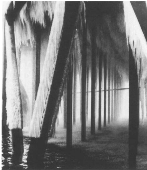
Figure 34.15 Ice on natural-draft tower (no de-icing ring fitted)
