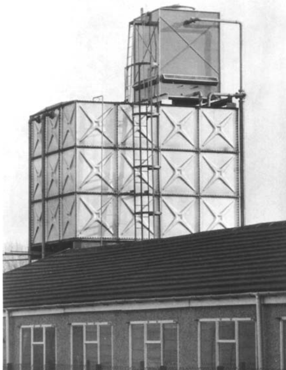
Figure 34.13 Cyclic heat load using small tower and large water storage. This is a good idea and sound engineering, but the access panel is on the wrong side (30 ft drop to ground level)
