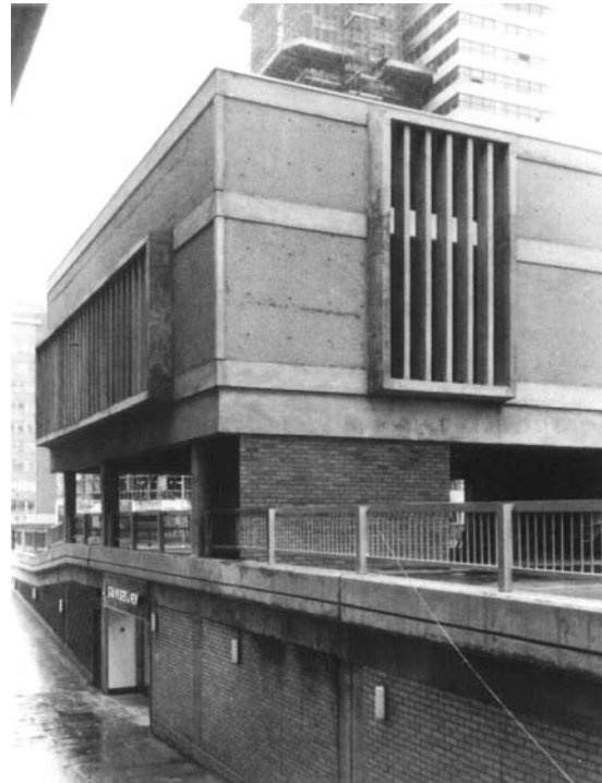
Figure 34.6 Cooling plant, including towers, installed as a separate unit on a supermarket satisfies the architect, town planners and the end-user
