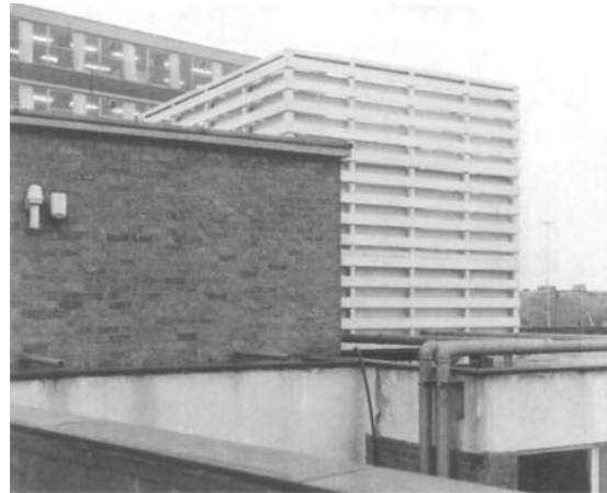
Figure 34.14 An attempt to conceal tower and reduce noise, resulting in starvation of air and failure in performance
