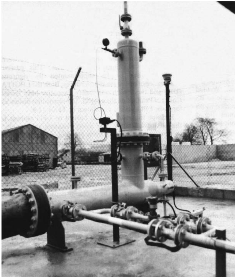
Figure 20.6 Hot-water heated LPG vaporizers. (Courtesy of Esso Petroleum Co. Ltd)
