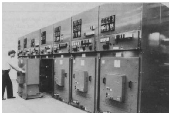
Figure 16.2 NEI Reyrolle SF 6 switchgear
