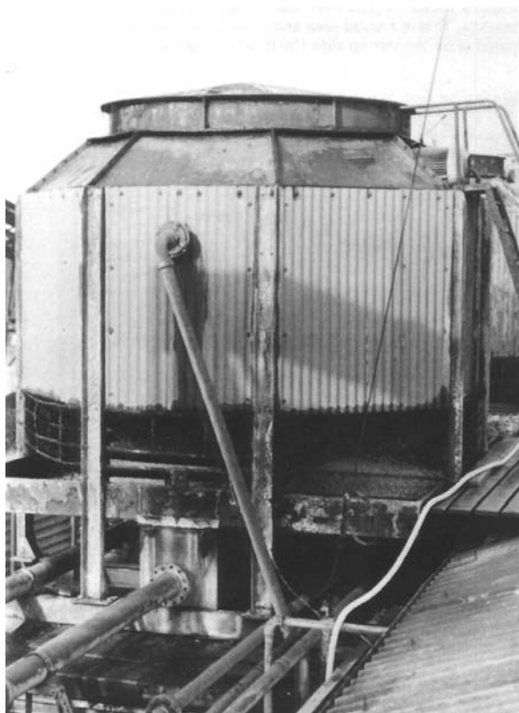
Figure 34.16 The effects of corrosion. Structural failure is visible (holes in fan casing)
