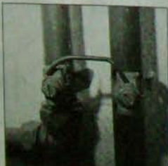
Copper water supply pipes earth bonded with a length of copper wire, fixed between a pair of earth clamps.
