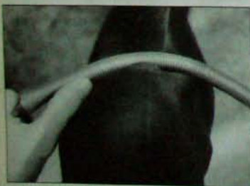
Bending 10mm copper tubing around the knee inside a spring support to prevent kinking.
