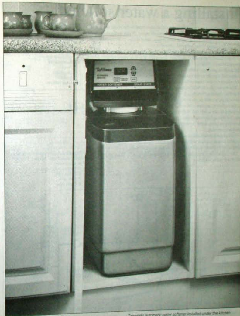
Tapworks automatic water softener installed under the kitchen worktop, where it is easily connected to the rising main.
