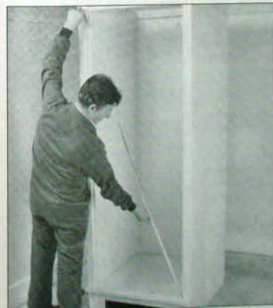
5 Check that the cubicle is square by taking diagonal measurements across the door opening. Both measurements should be the same; if not, adjust the panels until they are. Then tighten the screws in the sequence specified.
