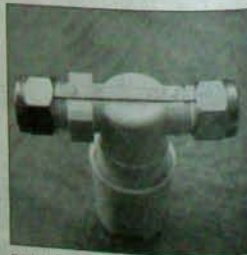
Earth bonding copper strip built into a plastic shower stoptop. The compression nuts are of plated brass.
