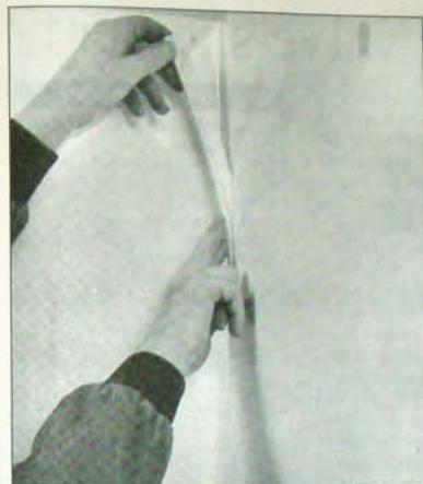
3 Lengths of flexible sealing strip are fitted between the walls to provide waterproof joints. The strips can simply be pressed into the gaps between the loosely-assembled panels with your fingers. Make sure they are seated correctly.
