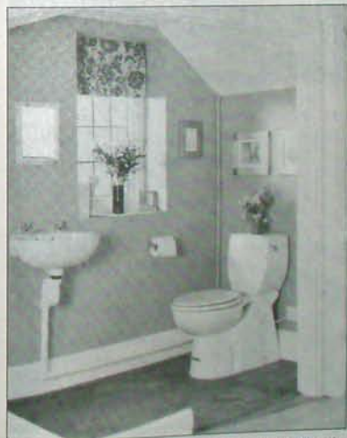
This demonstrates what can be done with an understairs cupboard, in this case using the Sanichasse from Saniflo, which incorporates the macerator unit within the WC pan.
