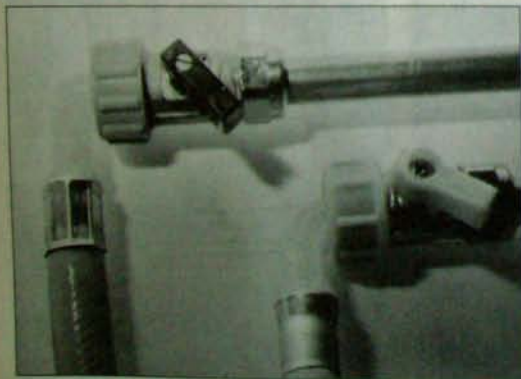
Modern washing machines need a hot and cold fill, which means extending the pipework, as in this case, or tapping into existing pipework and fitting the appropriate servicing valves so that the water supply to the machine can be turned off when not required. The washing machine hoses simply screw onto the valves hand-tight.
