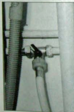
For the cold-fill dishwasher, the supply is fed from an existing cold water pipe, using a compression fitting that also incorporates the service valve.
