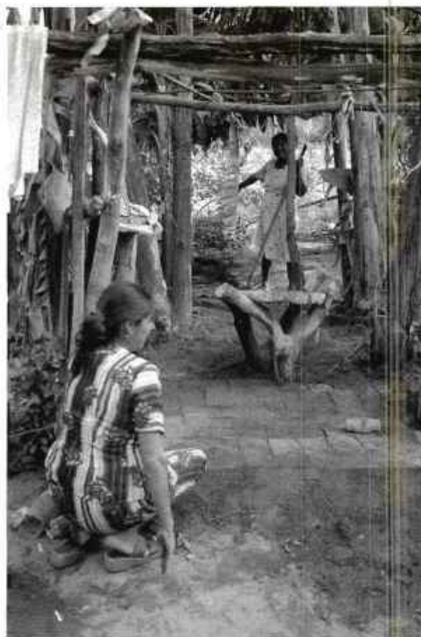
Garden committee members installing a masonry floor (normally men's work) over the puddle that a neighbor used to stand in while doing laundry.
