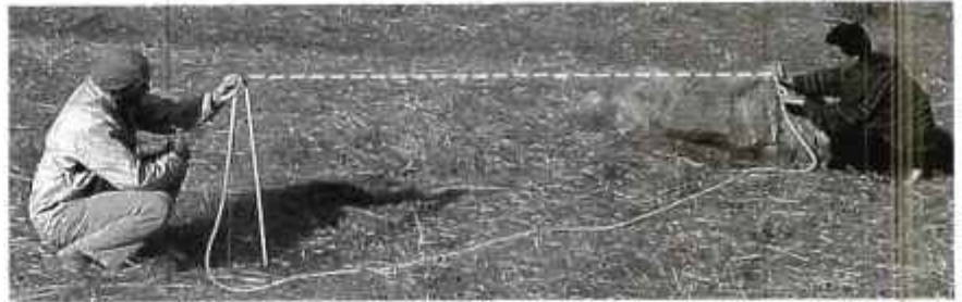
Checking levels with a water level. Person at right adjusts tube until water level is at her reference mark. Person at left measures from water level in tube to ground.
