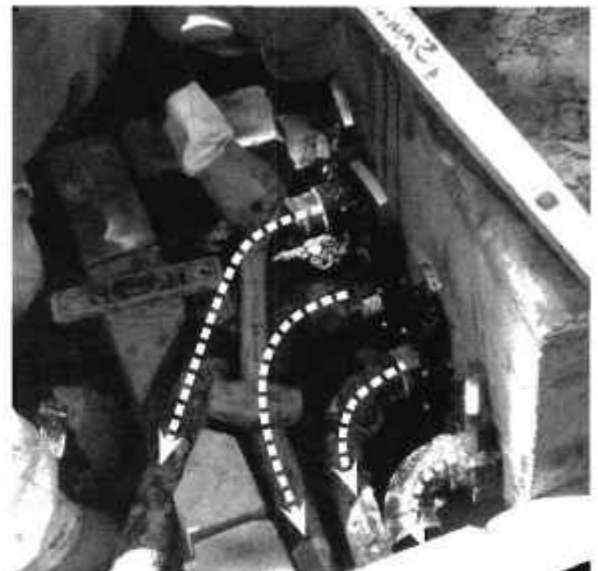
Dipper distribution box with a brick enclosure around individually valved outlets.
