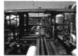
The competition: A seawater desalination plant provides some of the world's most costly, energy-intensive freshwater.
