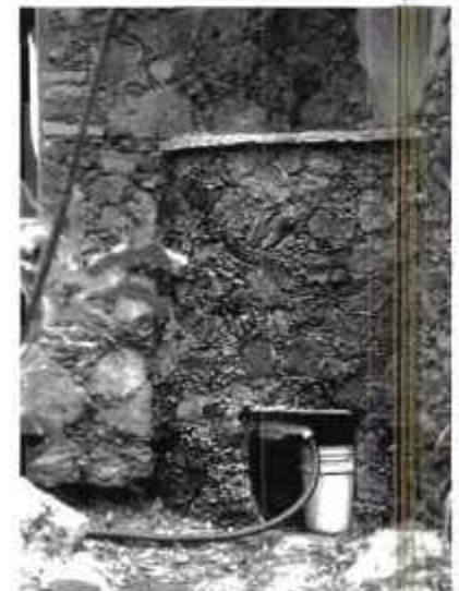
Multi-Mode Greywater Tank with enough fall to fill a bucket from a valve at the bottom. A quarter-cylinder shape, this tank fits nicely in an inside corner of the house. It holds 50 gal (190 L) and is made of ferrocement faced with stone. The floor slopes strongly toward the outlet, so it drains completely of water and is self-cleaning of solids.
