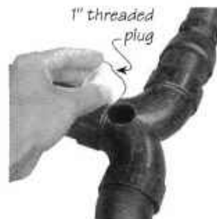
A double ell retrofitted with inspection access. The access is sealed with a threaded plug. 49
