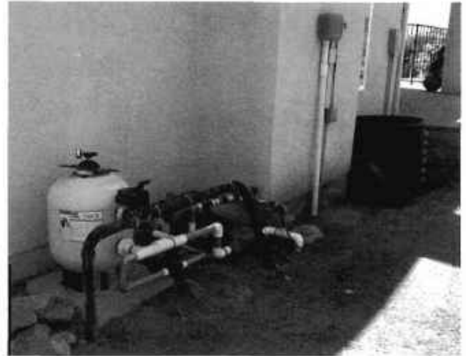
ReWater surge tank, sand filter.
