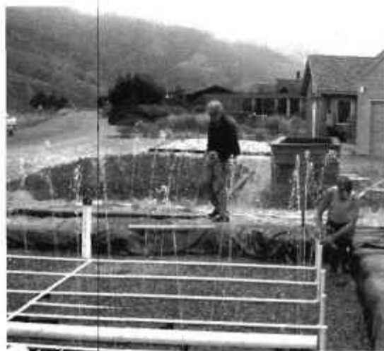
Orenco sand filter system being pressure tested in Stinson Beach, CA. The pipes will be covered with sand and plants. These houses are on a narrow sandbar with ocean on one side and an estuary on the other. As part of one of the most stringent monitoring programs in the country, Stinson Beach inspects all on-site wastewater treatment systems annually.
