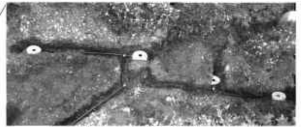
Four outlets with 1/4 each of bath/shower flow. These subsurface outlet chambers are way undersized. The owner plans to replace them with a continuous row of infiltrators 30' (10 m) long and 14" (35 cm) wide.
