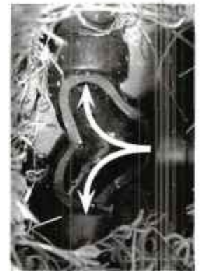
Cutaway view of a double ell, a flow-splitting fitting that is largely self-cleaning with no filtration. This one is part of the first known Branched Drain network. I valiantly tried to clog it with pure kitchen sink water—took the sink strainer out and pushed bowls of soggy granola and pot scrapings down the pipe for half a year. The p-trap clogged every other day, but the Branched Drain network never did.
