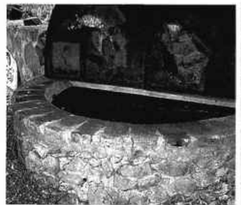
Beautifully made but ill-conceived greywater storage tank. This 250 gal (1 m 3 ) tank is the final of a four-chamber system that converts greywater to blackwater over the course of a week. The blackwater smells wicked, and generates hydrogen sulfide, which has eaten through the steel lid.
