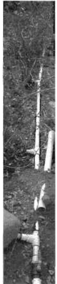
An exception: "Twisted tees" system in Santa Fe, NM has been successfully tuned so that the same amount of laundry water comes out each outlet, which branch off progressively lower until the end.
