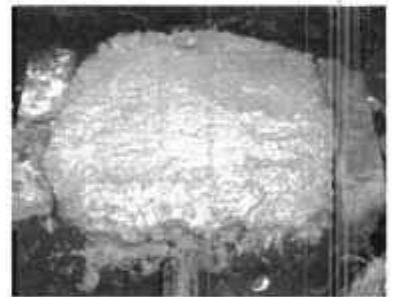
A pad of stiff concrete mix held in place by bricks awaits the dipper.
