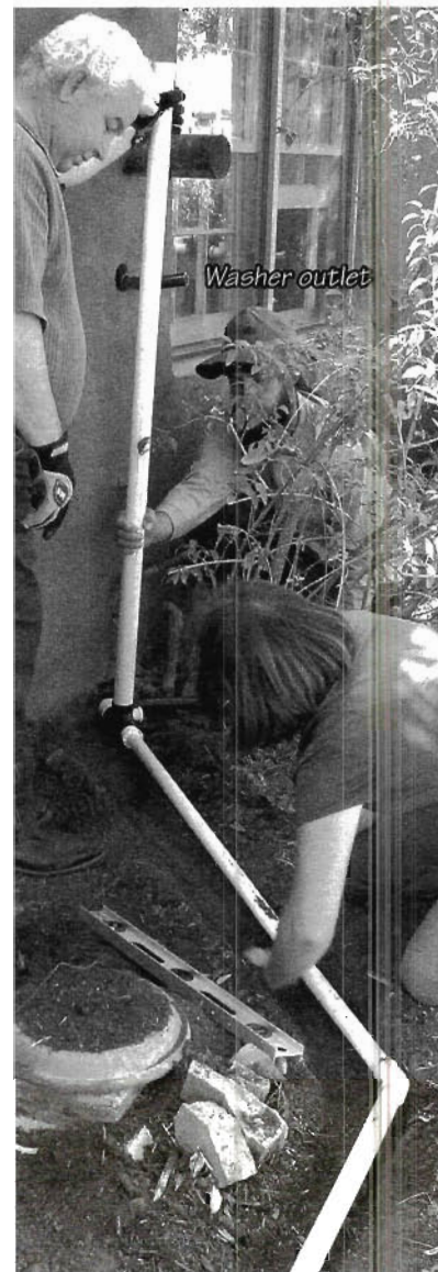
Leveling a Drumless Laundry line buried 4" deep in a hard-freeze climate. This line ran fine all winter, even though the plumbing inside the house froze!
