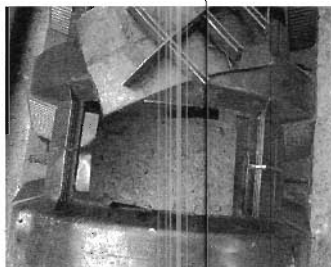
Making a lid, access port: Cut out a section between structural ribs with a sawsall or keyhole saw.
