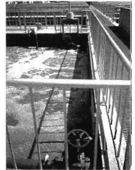
An activated sludge sewage treatment plant dumps greywater in the ocean after energy- and chemical-intensive treatment.
