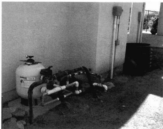
ReWater surge tank, sand filter.
