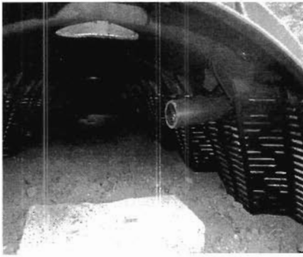
Infiltrator, inside view.
