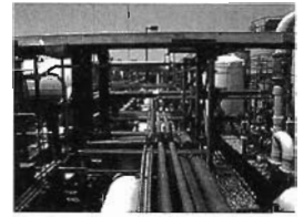
The competition: A seawater desalination plant provides some of the world's most costly, energy-intensive freshwater.
