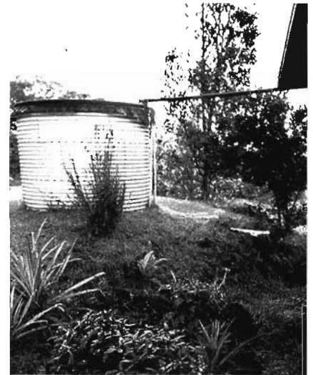
Rainwater harvesting provides all domestic water by gravity for a house near Hilo, HI.
