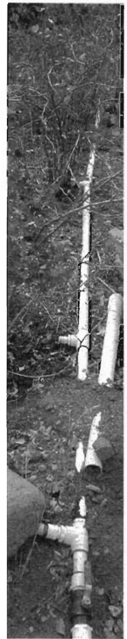
An exception: "Twisted tees" system in Santa Fe, NM has been successfully tuned so that the same amount of laundry water comes out each outlet, which branch off progressively lower until the end.
