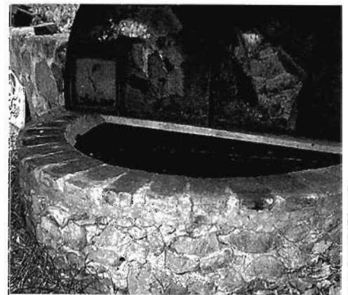
Beautifully made but ill-conceived greywater storage tank. This 250 gal (1 m 3 ) tank is the final of a four-chamber system that converts greywater to blackwater over the course of a week. The blackwater smells wicked, and generates hydrogen sulfide, which has eaten through the steel lid.
