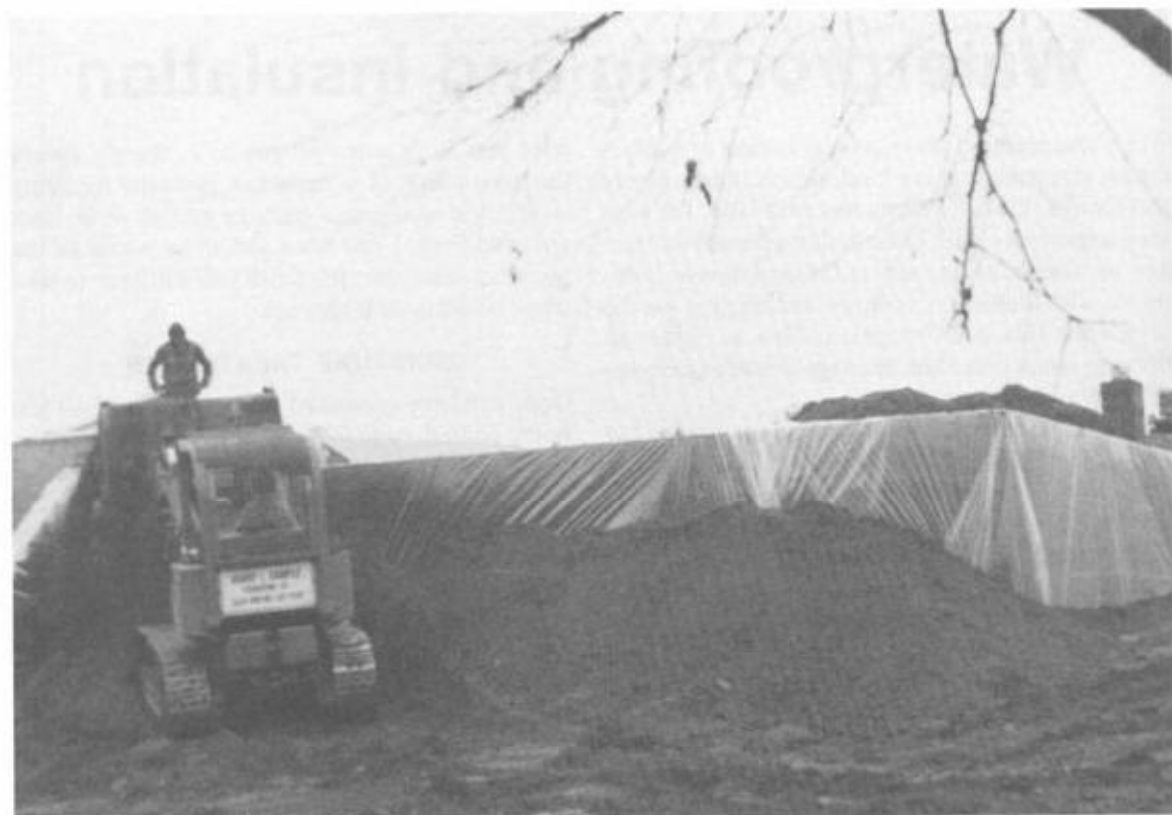
Fig. 11-1. The structure was coated with two coats of hot tar and then wrapped in 6 mil polysheets.
