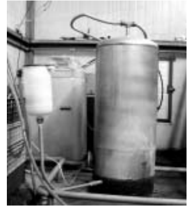
Figure 17. Electric boiler to feed steam into the bags in bulk.
