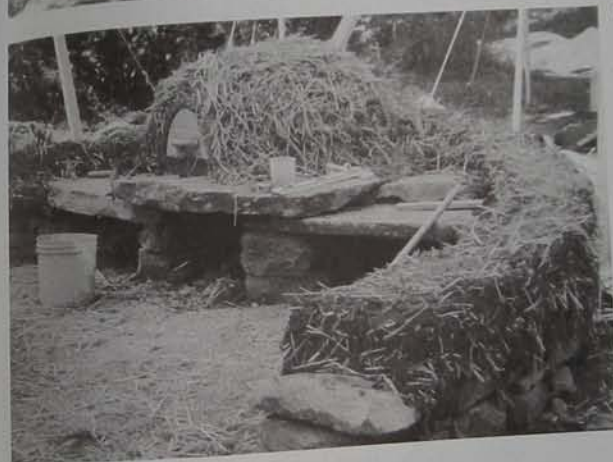
COMPLETED INSULATION LAYER Awaiting finish plaster. Note the massive foundation. This oven was built in New York state, where flagstone is abundant.
