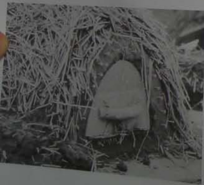
DETAIL—DOOR OPENING & BAKING DOOR Easier to fit the door at this stage, and then build on accordingly. The nails provide a "key" to help bond the next layer of cob.
