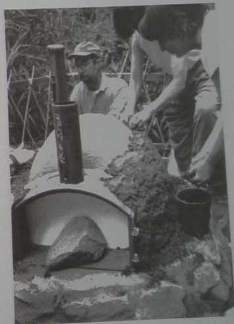
NOTE THE CUSTOM-MADE, WELDED STEEL DOORFRAME AND CHIMNEY The rock is leaning against a piece of cardboard, which is keeping the sand form from falling out of the open door (photo courtesy of N. Waddoups)
