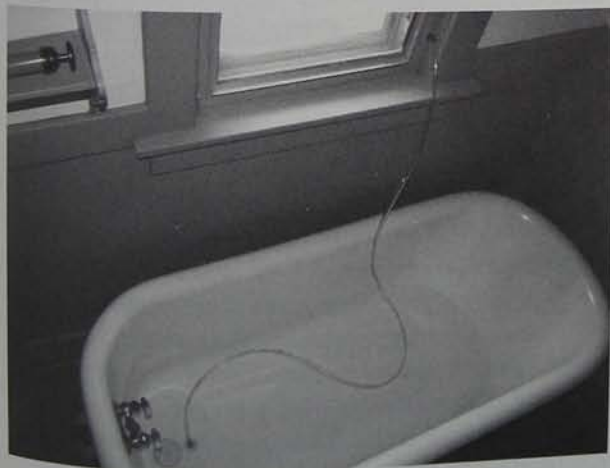
Fig. 4.28A. Vinyl tube suction-cupped to bottom of tub and run through window frame accesses greywater for landscape use and bypasses having to deal with otherwise inaccessible tub drain plumbing. Note that this type of system may not seem convenient, although it may be a useful option for otherwise inaccessible greywater.
