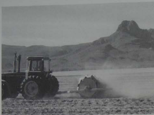
Fig. 3.13A. An imprinter roller pulled by a tractor creating and seeding imprints on barren, compacted earth, Marana, Arizona
