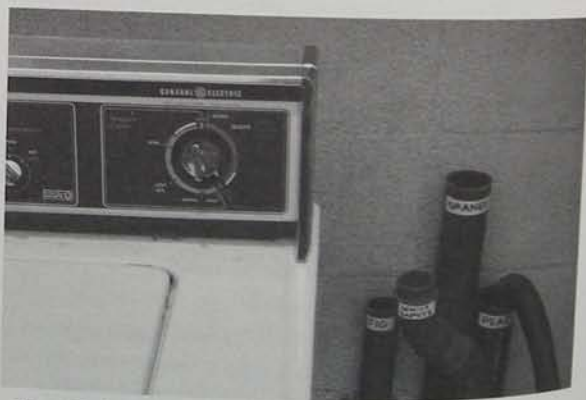
Fig. 4.26. Greywater drains (marked with destination; fig, white sapote, orange, and peach) beside washing machine. Drain hose from washer is placed in a different pipe with every load of laundry. An option for households occasionally using non-biocompatible detergents is to include an additional marked drainpipe going to the sewer.
