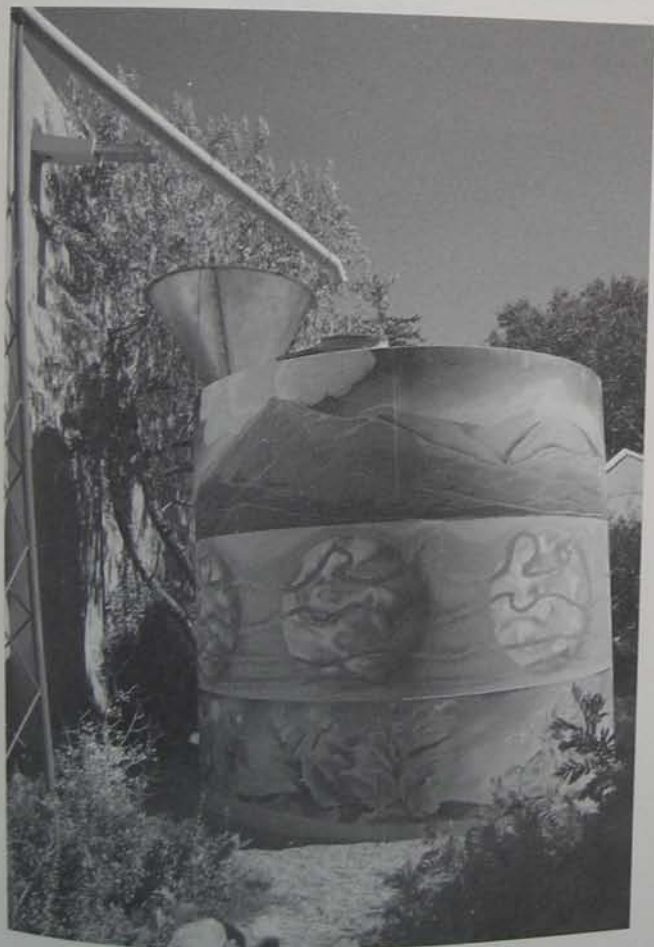
Fig. 3.31. A 10,000 gallon (38,000 liter) steel tank/mural and dry system downspout collecting roof runoff for irrigation, Children's Museum, Santa Fe, New Mexico
