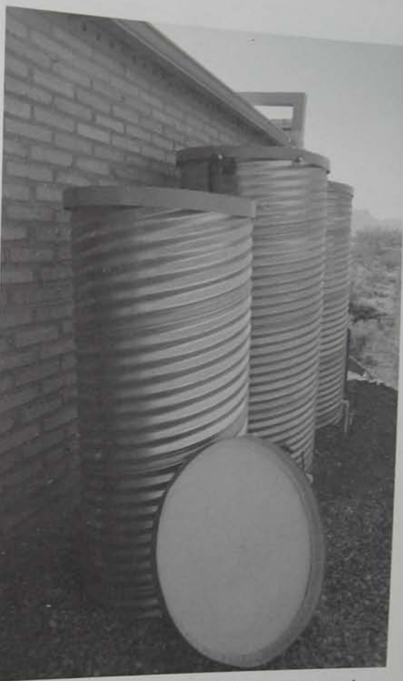
Fig. 3.32. Culvert tanks with light-, insect-, and critter-proof lids. Overflow moves from one tank to the next, then out to vegetated basins not shown. Milagro Cohousing, Tucson, Arizona
