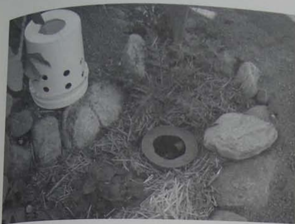
Fig. 4.27. Each greywater drain outlet is placed in a mulched and vegetated infiltration basin that also harvests rainwater and runoff. The drain pipe empties into an upside down bucket with holes in the sides, creating a chamber of air into which roots will not grow, so the pipe will not clog. An example bucket chamber sits beside the basin so you have a better idea of what the bucket within the basin looks like. Ordinarily the flat rock beside the drain outlet is placed over the outlet to keep the greywater below the surface of the rock and mulch. The rock lining the basin stabilizes the basin's edge.
