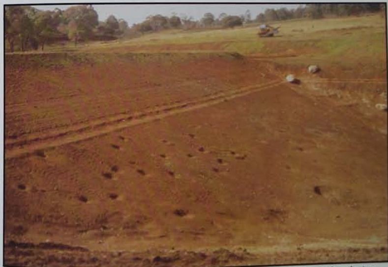
Plate 58 Emptied dam of Plate 77. Wave action from two days of explosive treatment caused the two lines across the wall. Below the lines, the pockmarks show where the various charges exploded. The dam leaks down through the mudstone excavation area and not through the wall.
