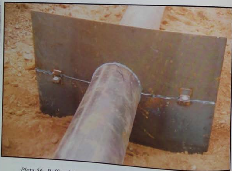
Plate 56 Baffle plates prevent water from flowing along the outside of the pipe. They are bolted in place. The use of a sealing compound around the pipe and between the baffle plate halves prevents seepage.
