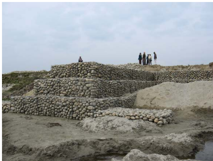
Figure 4: A newly constructed spur shown before the monsoon. The base of the river and the spur apron are clearly visible in the dry season. Photo: Practical Action Nepal.
