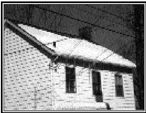
HOUSE WITHOUT PROPER VENTING
