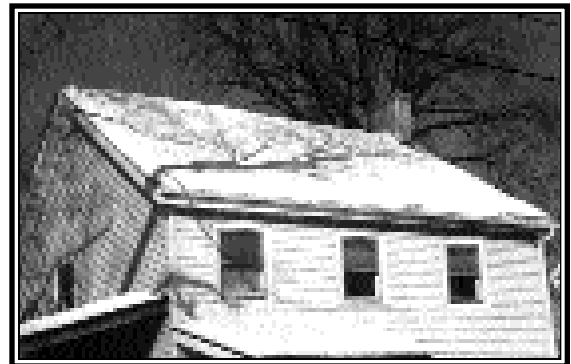
HOUSE WITH PROPER VENTING
