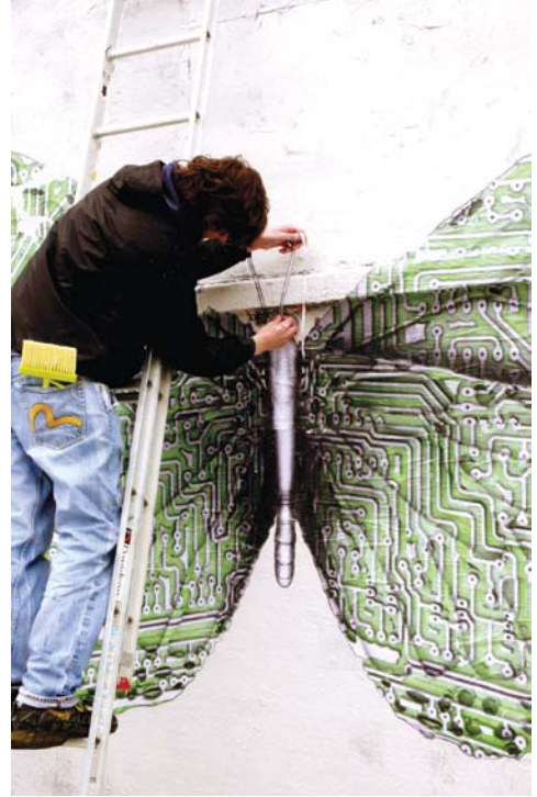
3.22 Ludo installing a circuitry butterfly on a building wall in Brooklyn. Photo by Jaime Rojo.
