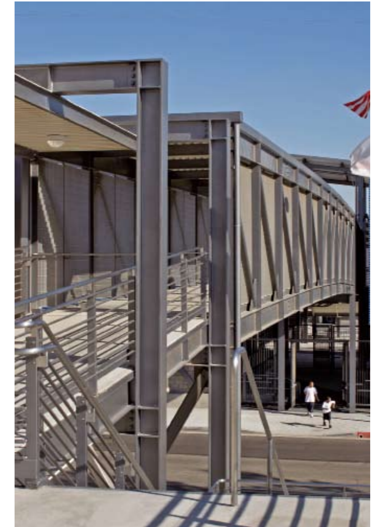
Durable, low-maintenance materials were used throughout the design
