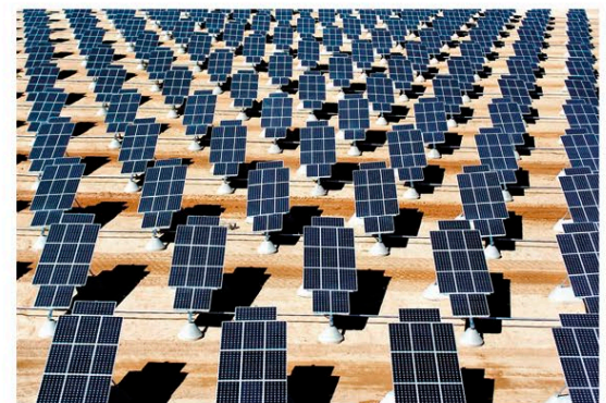
▽ Catching the sun Around 70,000 solar panels in the Nevada Desert provide 25 percent of the power used at the Nellis Air Force Base. It is the largest solar power plant in the western hemisphere; such projects are held up as models for renewable energy.
