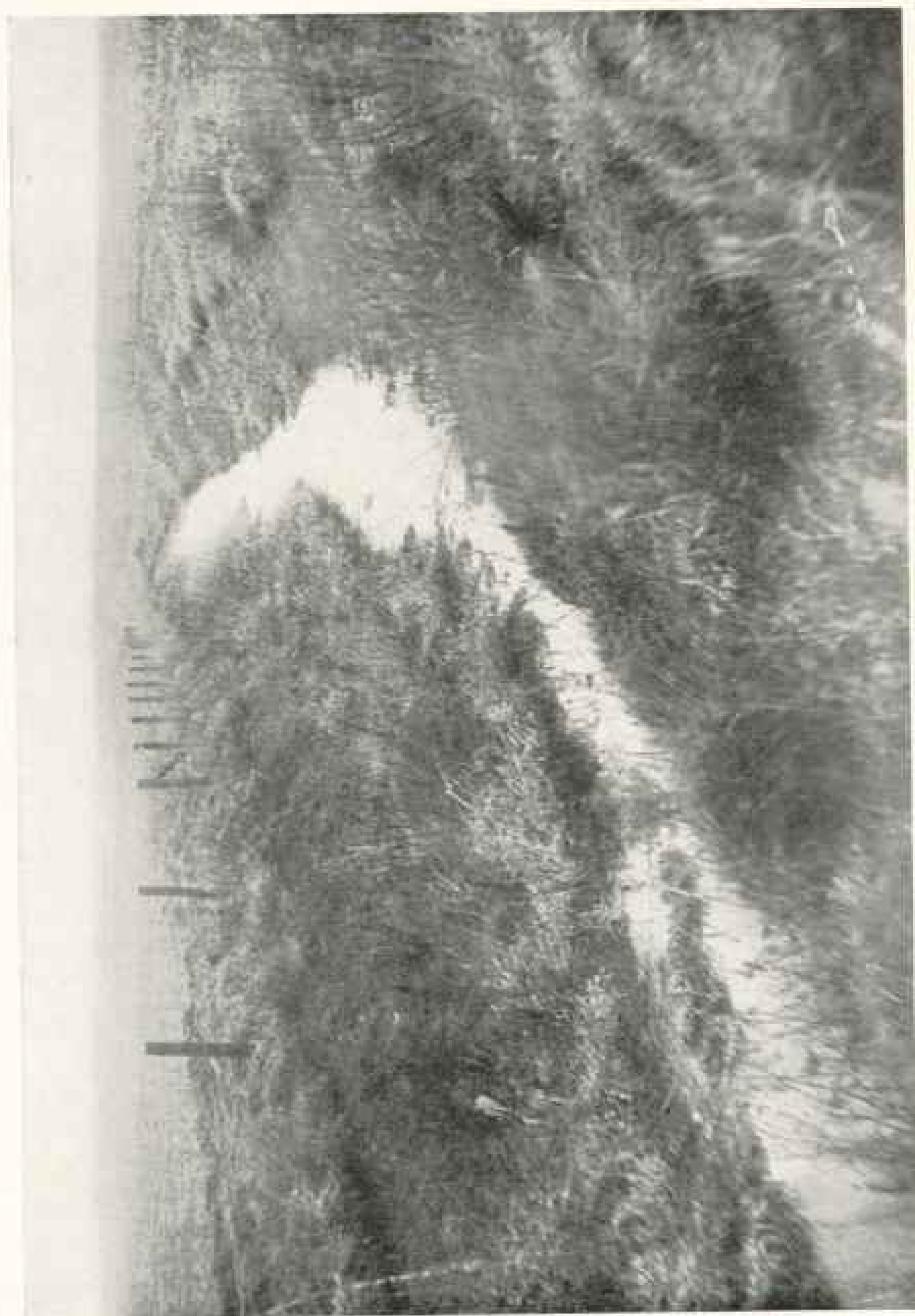
A POORLY CONSTRUCTED DRAINAGE DITCH—SIDES CAVED AND ERODED
