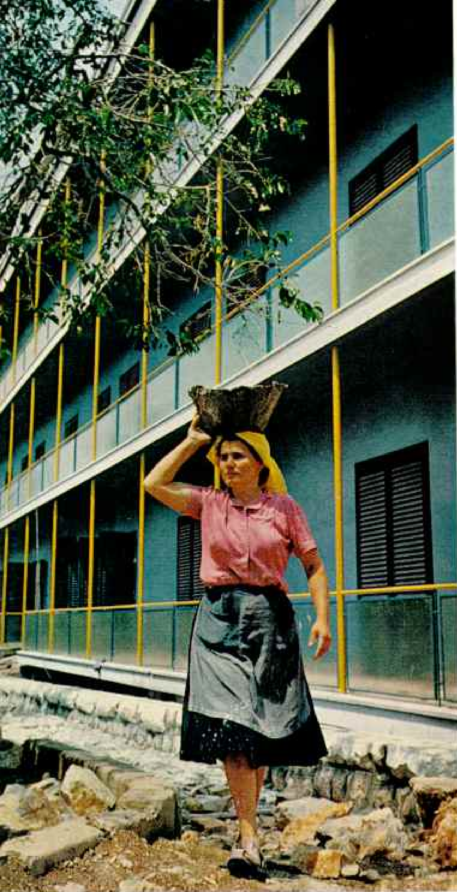
Old methods, new architecture: Shuttling headloads of plaster into an apartment building nearing completion, this Šibenik worker, like many Yugoslav women, helps relieve the housing shortage.
