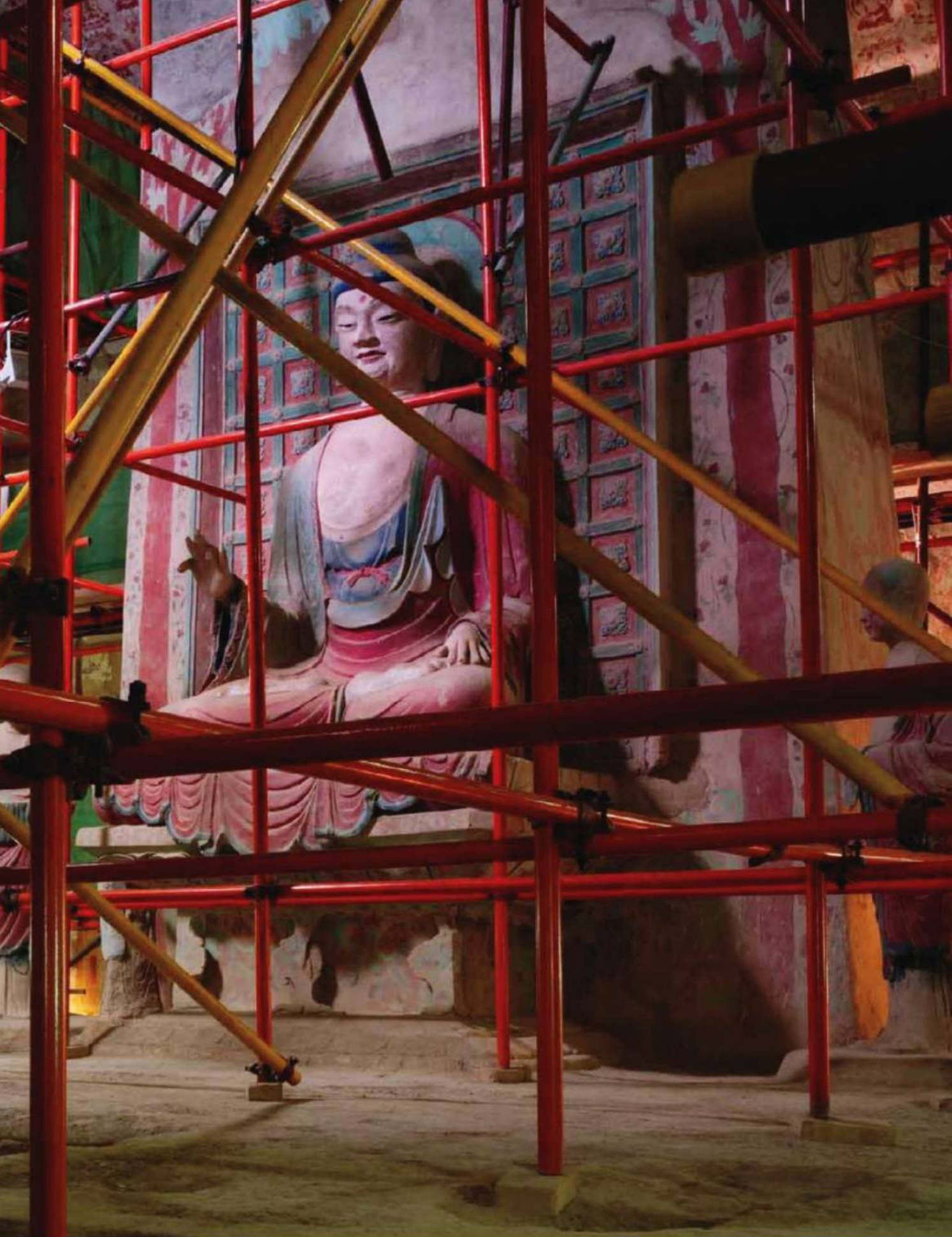
Scaffolding rises in a tenth-century grotto, part of a conservation effort to stave off the effects of sand, salt, soot—and the damp breath of tourists.
