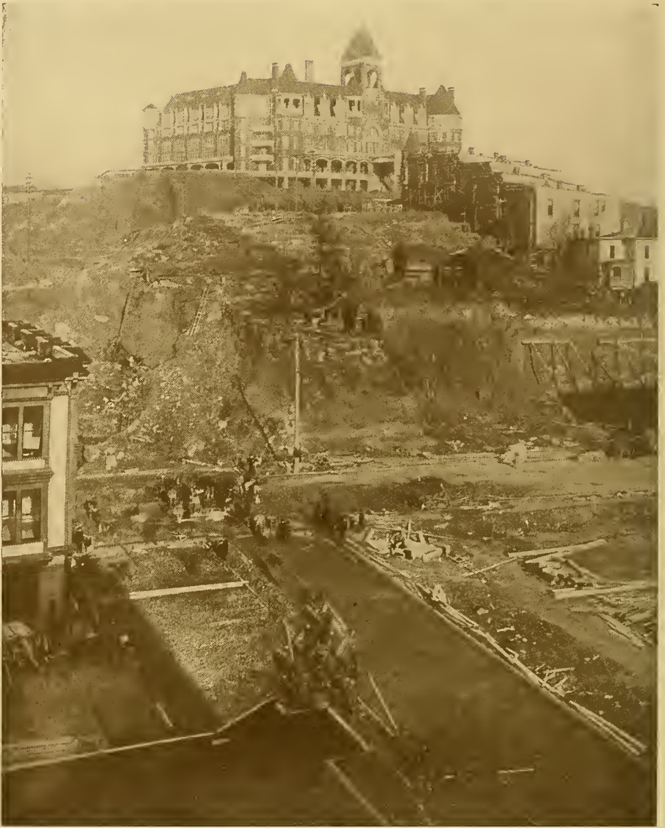
This and the succeeding three pictures show what is being done in Seattle in the way of removing hills for the expanding business district. These regrading projects involve the removal of more dirt than any other modern enterprise outside of the Panama Canal. The total depth of the excavation, from the foundation of the Old Washington Hotel, shown in this view, to the foundation of the New Washington, was 108 feet.
