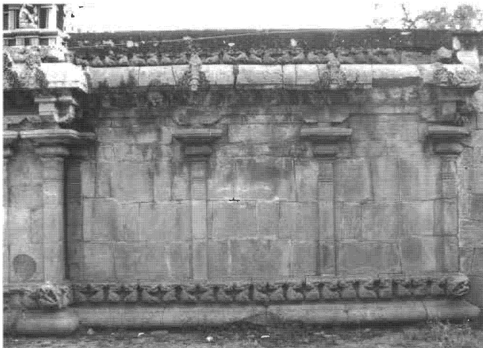
Fig. 4. South wall of the ardhamandapa , Candraśekhara temple, Tiruccendurai. Note the basement moldings below the pilastered wall surfaces and the entablature above. Roughly cut stone blocks just visible at the far right are part of a later addition to the front of Naṅgai's temple.
