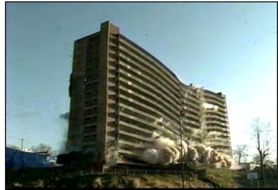
Classic building crimp from demolitions
