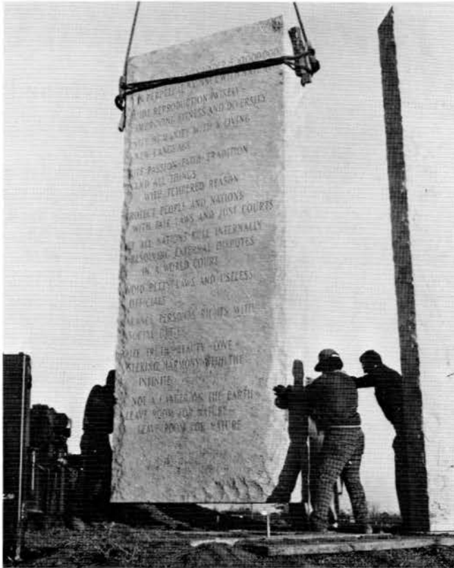
"Ever so gently!" describes how the crane and setting crew handled the stone sections and their enormous weight. As shown above, stainless steel dowel pins were placed in each of the granite bases and the upright sections were set on the pins.
