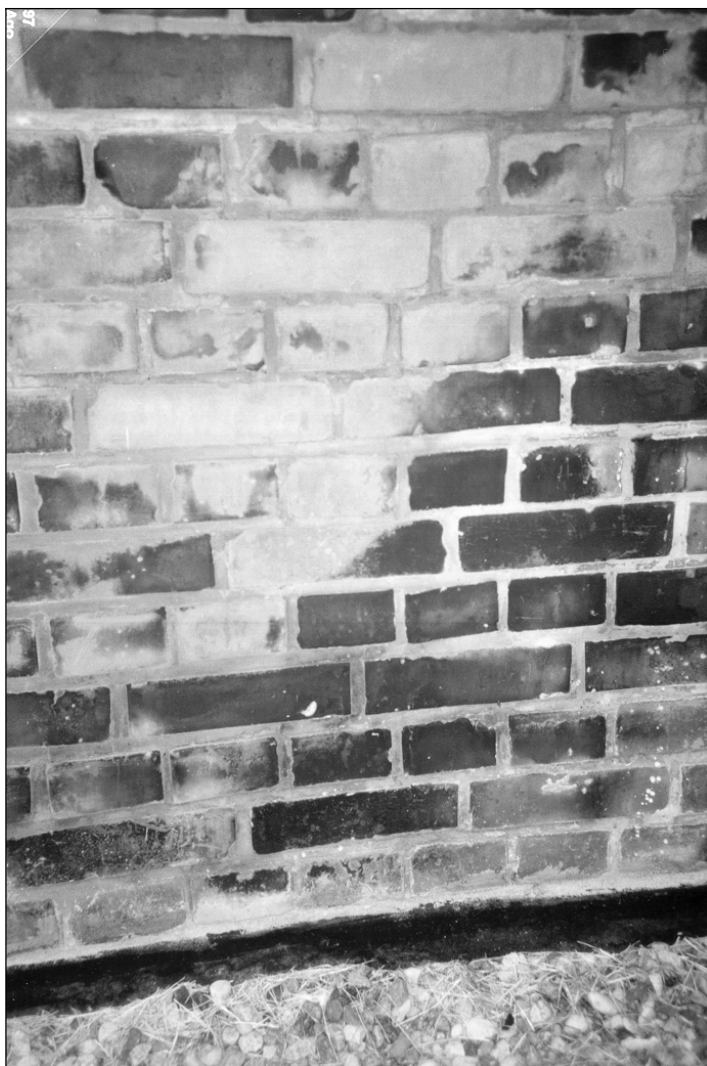
Photo 15: Delousing chamber at Stutthof, east side, exterior. The brick exhibits the typical blue pigmentation caused by iron cyanide. © Carlo Mattogno
