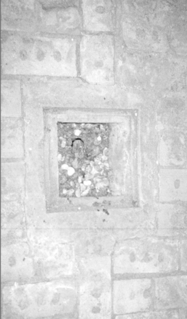
Photo 12: Delousing chamber at Stutthof, interior. Drainage shaft in the middle of the brick floor underneath the Zyklon B introduction hatch. © Carlo Mattoño
