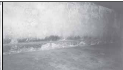
Fig. 41: Blue staining of the Zyklon B disinfestation installation, east wall of chamber III of barrack 41 in Majdanek camp. (© C. Mattogno 202 )
