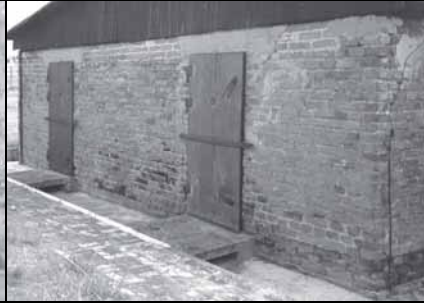
Fig. 43: Blue staining of the Zyklon B disinfestation installation, chambers II and III (exterior wall), of barrack 41 in Majdanek camp. (© Carlo Mattogno 203 )
