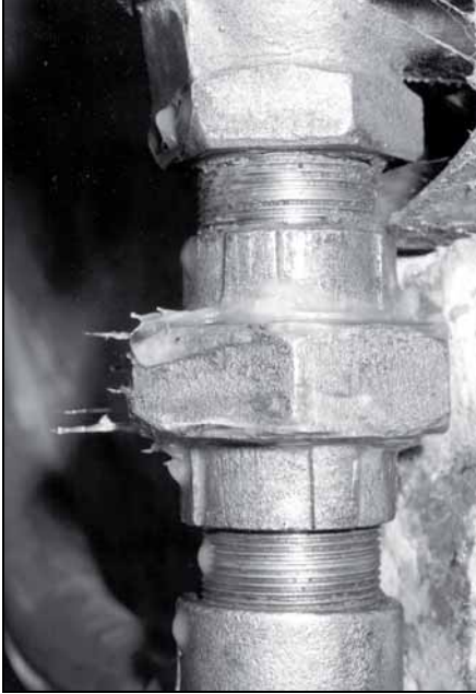
Fig. 92: Closeup of plumbing underneath the gas chamber covered in vaseline to indicate leaks.
