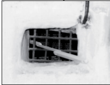
Fig. 33: Opening with grate in the wall of room I in the disinfestation wing of building 41, Majdanek (see Fig. 31)
