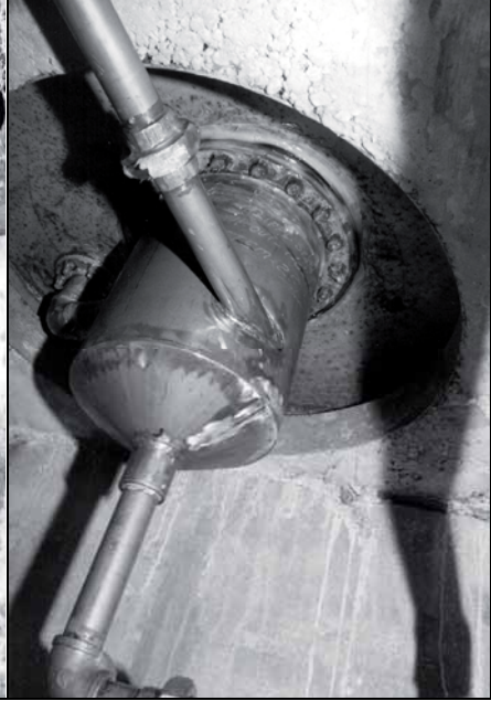
Fig. 93: View of stainless steel plumbing and chemical container directly under seat in gas chamber.
