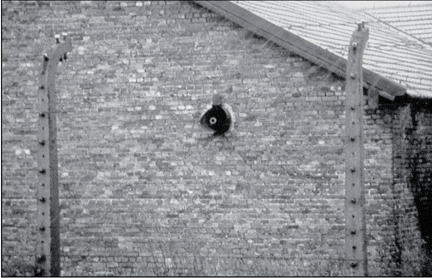
Fig. 24: One of the two ventilation outlets from the disinfestation wing of building BW 5b, without equipment today. The other is located on the same wall slightly to the left. The end of a water pipe put in there after the war is visible.
