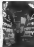
A worker is seen in the foreground as the Reichstag is reconstructed in Berlin.
