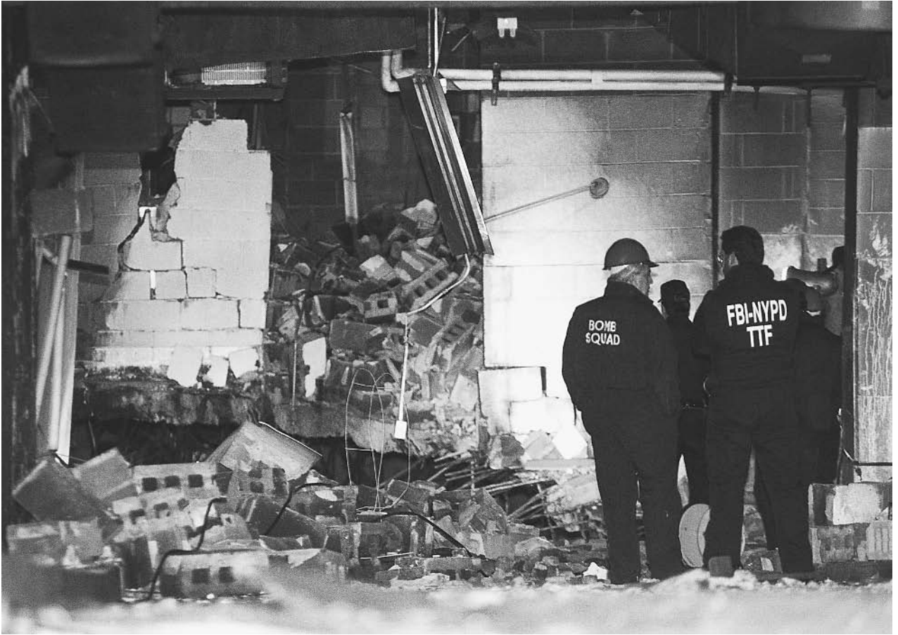
FBI agents view the damage caused by the 1993 terrorist bombing of the parking garage at the World Trade Center towers in New York. ©REUTERS NEWMEDIA INC./CORBIS.
