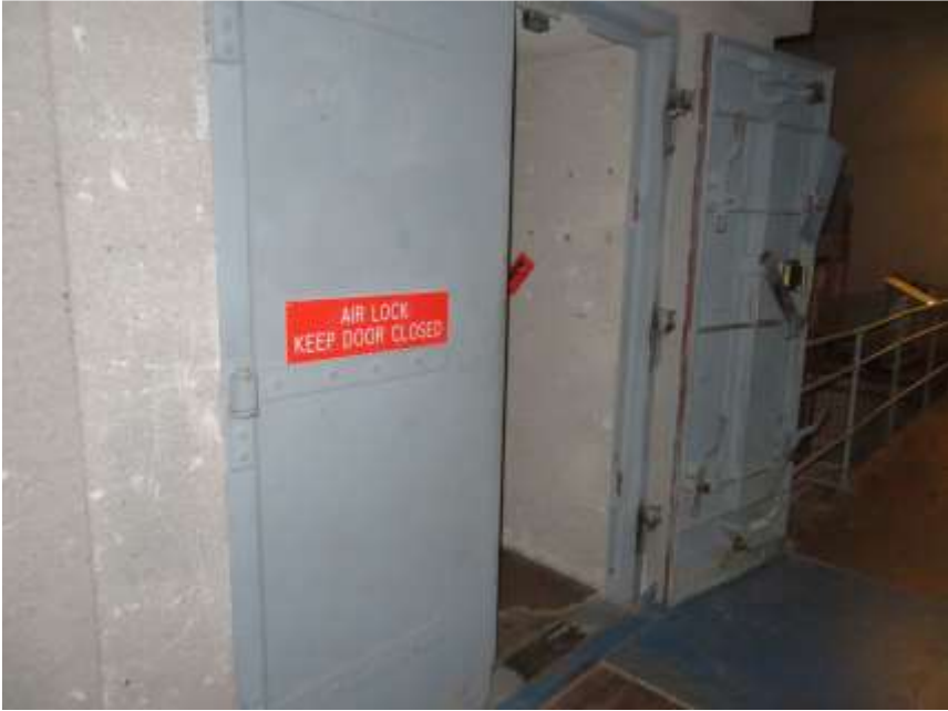
One of the doors which was meant to help keep out radiation/fallout following a nuclear attack. (Photo by Andrew Johnson – 2018)
