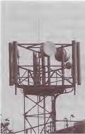
Figure 235: This abomination is on the roof of Cowes High School on the Isle of Wight with children and staff sitting under it day after day
