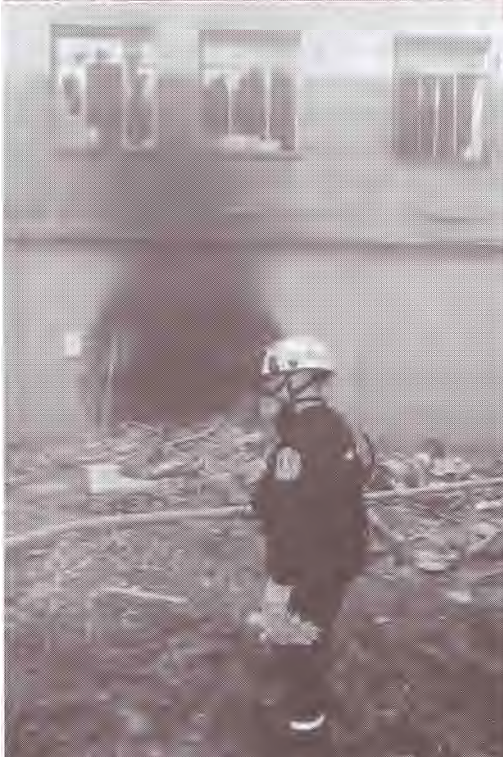
Figure 178: ... This hole, some nine feet across, is 310 feet and three rings of heavily reinforced walls away from the impact point
