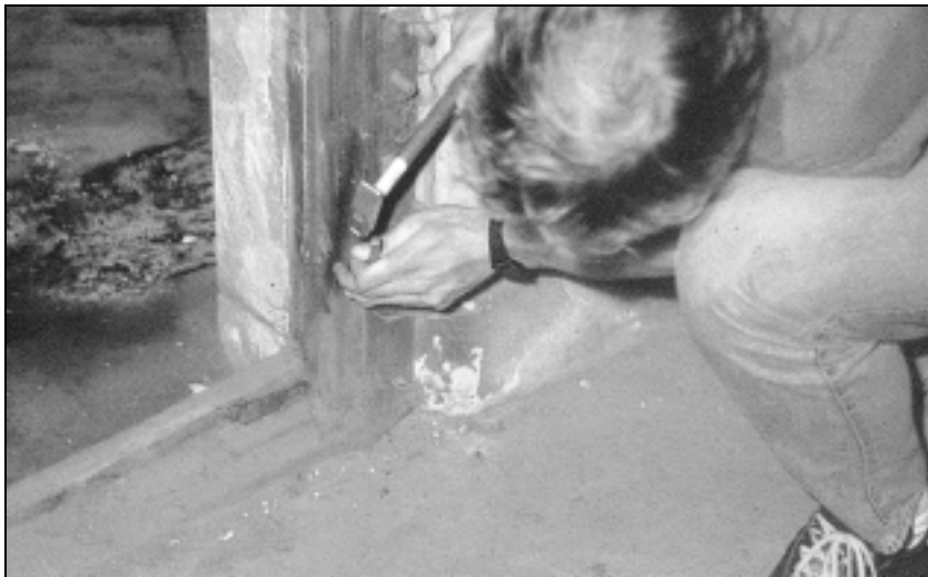
Fig. 70: Picture of the door frame in disinfestation wing of building 5a. the lower, rusty hinge has developed Iron Blue under the influence of hydrogen cyanide. Sample taking location of sample no. 18.
