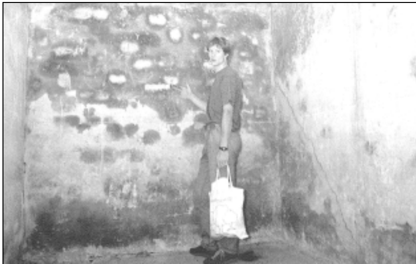
Fig. 69: Picture of a room located in the northwest of the disinfestation wing of building 5a (see Figure 18). The exterior walls are located in the background and to the right, showing intensive blue discolorations caused by iron Blue. Taking locations of samples 9 and 11 are visible. On the left in the picture is the interior wall, erected during the conversion to a hot air disinfestation chamber. Sample 10, with a slightly positive cyanide content, was taken from this wall.
