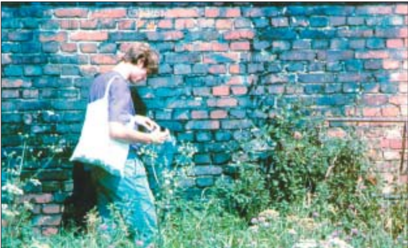
Color Image 2: Exterior southwest wall of the Zyklon B disinfestation wing of BW 5b in the Auschwitz-Birkenau camp: a deep blue discoloration, caused by cyanide compounds which penetrated the entire wall over the decades since WWII and formed the blue pigment with iron compounds contained in cement and bricks. This pigment is unaffected by 55 years of weathering.
