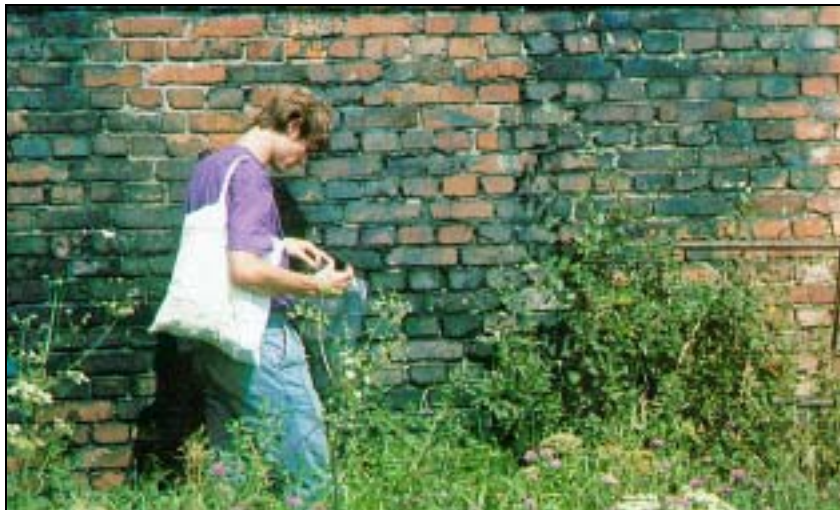
Fig. 71: In contrast to building 5a (see Fig. 68), the disinfestation wing of building 5b was used as a hydrogen cyanide delousing chamber for a longer period of time. Subsequently, the outside of its walls are covered with blue spots, unimpressed by 50 years of weathering here as well.
