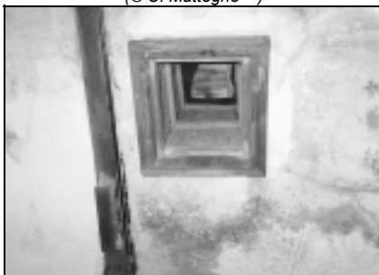
Fig. 63: Large Zyklon B disinfestation chamber, ceiling, barrack 41 in Majdanek camp. (© C. Mattogno 316 )
