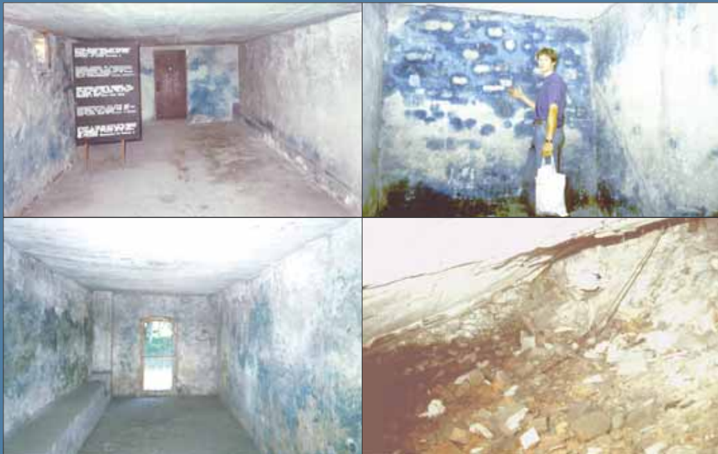
Blue staining of delousing chambers caused by Zyklon B: Majdanek (top left), Auschwitz-Birkenau (top right), Stutthof (bottom left). No such staining can be seen in morgue #1 (the alleged homicidal gas chamber) in crematory II at Auschwitz-Birkenau (bottom right).
