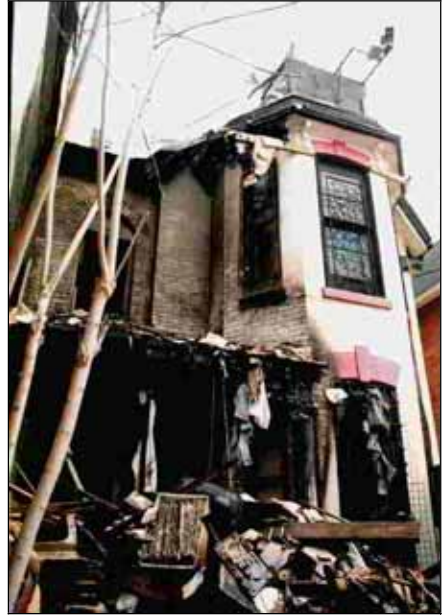
III. 154: Fire damage to the Zündel house after the arson attack on May 7, 1995.
