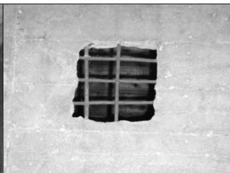
III. 102: Crematory Majdanek camp, alleged homicidal gas chamber, opening in the ceiling. © C. Mattogno
