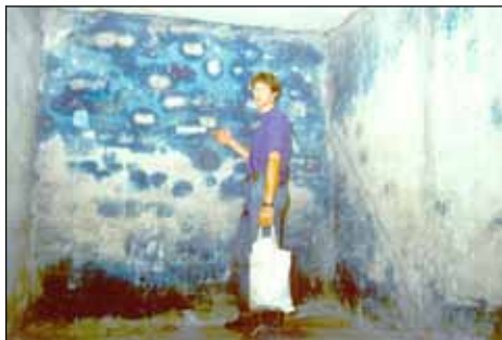
III. 54: Interior wall, northwest, of Zyklon B delousing wing of building BW 5a in Auschwitz-Birkenau.
