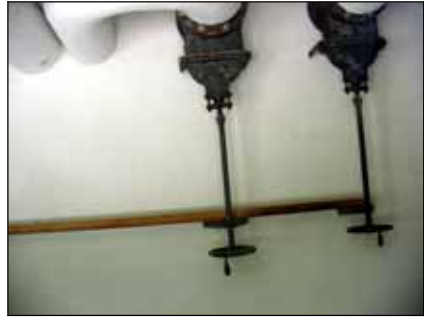
III. 10: Heavy insulated hot water (or steam?) pipes in the room behind the alleged gas chamber of Dachau camp, leading into the space above the current room. 122
