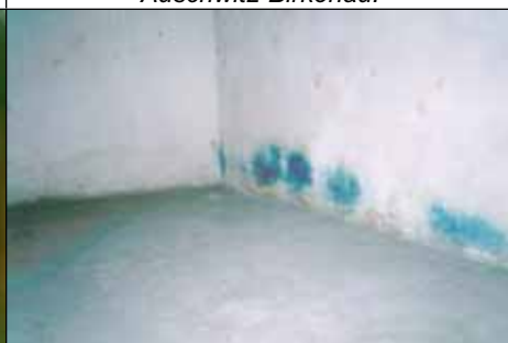
III. 57: Zyklon B delousing installation, chamber II (west wall), building 41 in Majdanek. (© C. Mattogno 523 )
