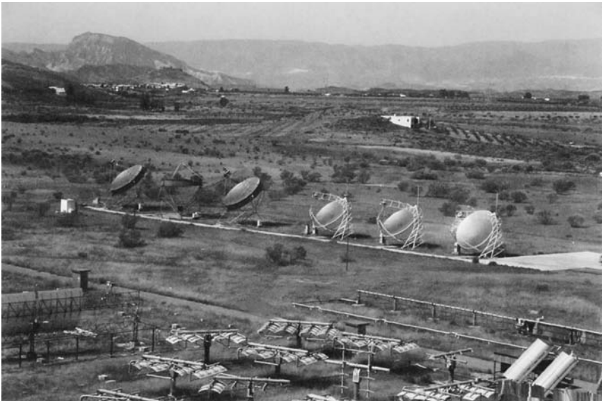
Each mirror in the array of cup-shaped mirrors automatically tracks the Sun and focuses the Sun's energy to heat water to makes steam. The steam is used to generate electricity. (Courtesy of the Sandia Laboratory, U.S. Department of Energy)
