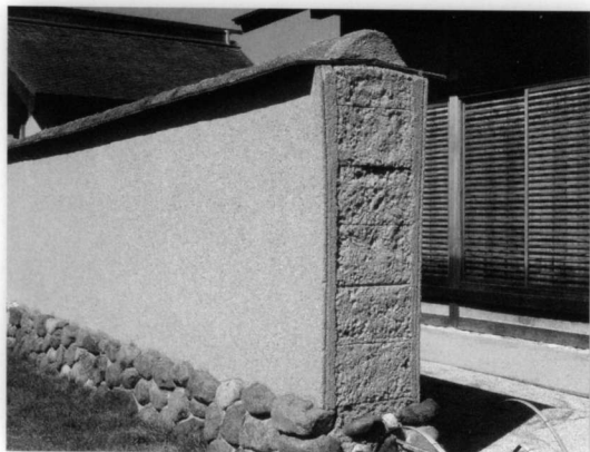
LEFT A cross section through the wall surrounding a samurai residence at Yuzuki Castle in Matsuyama. The different layers that have been added and rammed down can be clearly seen, as can the outer layer of rough plaster.
