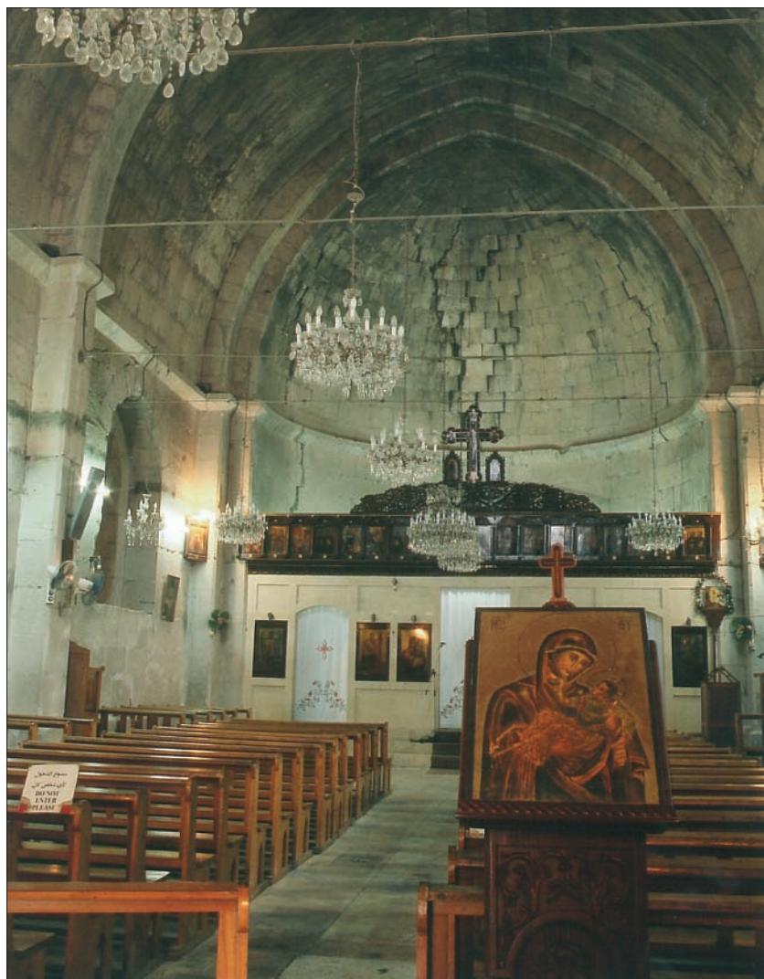
The lower part of the great fortified tower that rises over Safita (Castel Blanc) consisted of a church, which has remained to this day throughout the tumultuous history of Syria. The impact of earthquakes, which still sometimes rock this region, can be seen in the cracked semi-dome of the apse.
