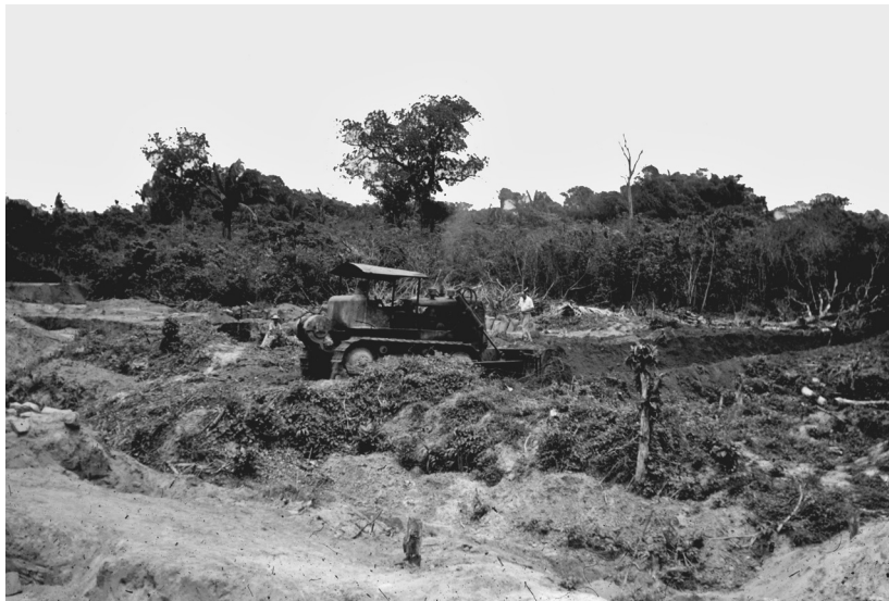
Fig. 7.1. La Venta, March 1955. An oil company bulldozer removes drift sand and 1942–1943 back-dirt piles from Complex A at the request of the archaeologists. National Anthropological Archives, Smithsonian Institution, ID number heizer_0304.
