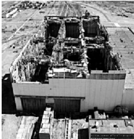
The collapsed roof of the MIK RN ( source: www.buran.ru ).
