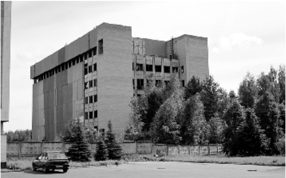
Due to the cancellation of the program, the largest Buran training facility in Star City was never completed and left to the elements (B. Vis).
