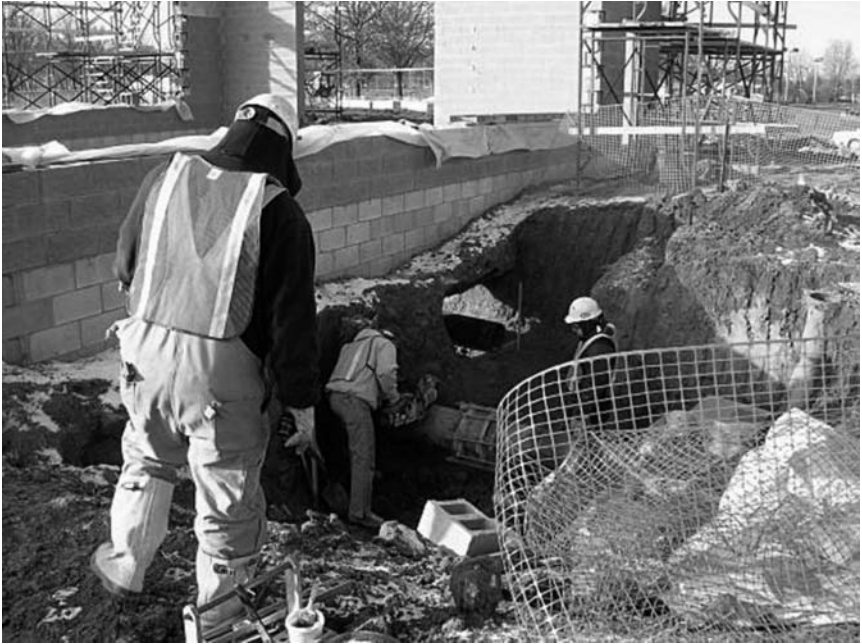
Belpre workers cut into a water main to create a bypass underneath the filtration plant.
