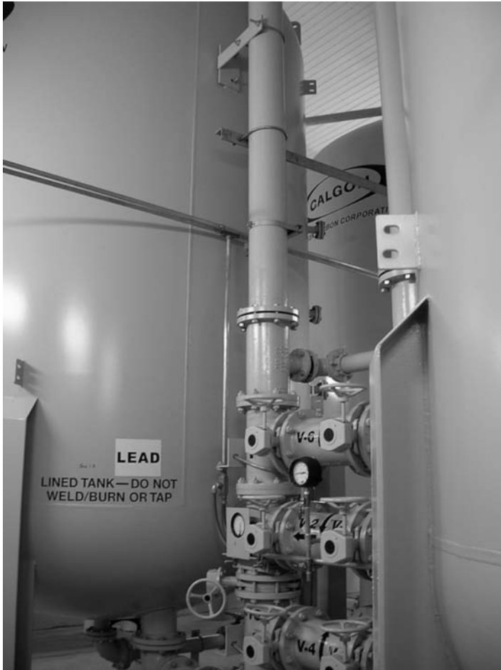
DuPont constructed this four tank granular activated carbon filtration system for the Tupper Plains Chester Water District.
