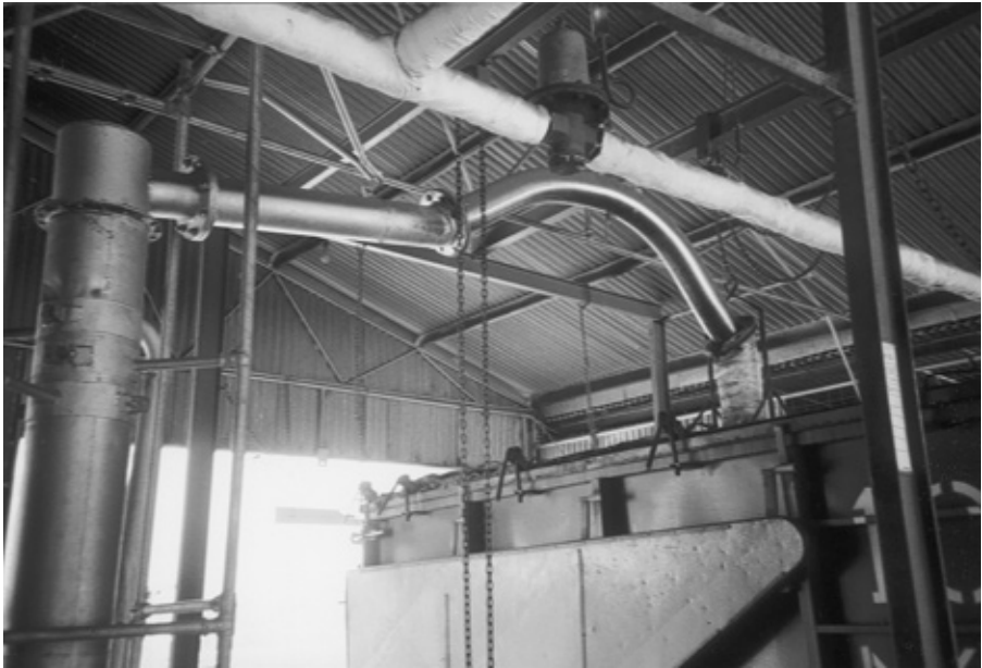
Figure 7.3 Trailer bin ready for distillation of Eucalyptus polybractea . Photo shows flexible duct which leads oil/water vapours from outlet at lid to multi-tubular condenser (photo: J. Coppen, courtesy of G.R. Davis Pty Ltd).
