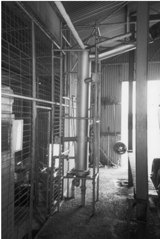
Figure 6.8 Multi-tubular condenser being used for eucalyptus oil distillation, Australia (photo: J. Coppen).
