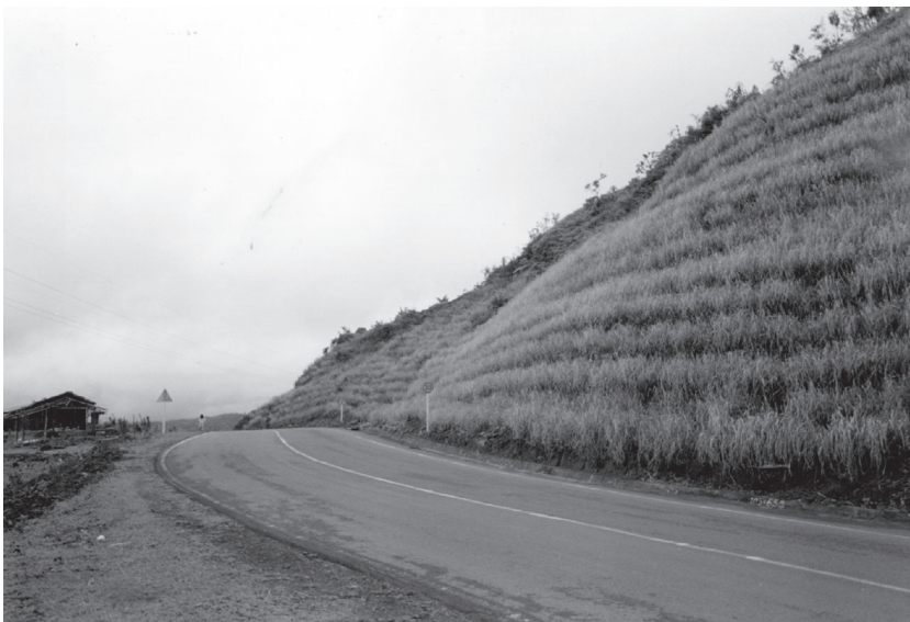
Figure 6.3 Vetiver Grass Technology is used as a bioengineering technique to stabilise this very steep cut batter of a road in the Philippines where landslides often occurred during the annual typhoon season. (Photo Credit: Noah Manarang).
