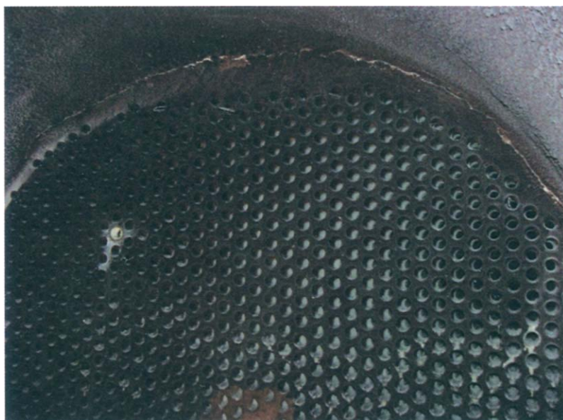
Fig. 3.4. Entrance to fire tube boiler tubes after Fig. 3.3's sulfur burning furnace. 1400 K gas (~11 volume% SO 2 , 10 volume% O 2 , 79 volume% N 2 ) leaves the furnace and enters the boiler. It turns 90° in the boiler and flows into the tubes. The tubes are surrounded by water. Heat is transferred from the hot gas to the water – cooling the gas and making (useful) steam. The tubes are typically 0.05 m diameter. Table 3.1 gives industrial furnace data. Sulfur furnace boilers are discussed by Roensch (2005).
