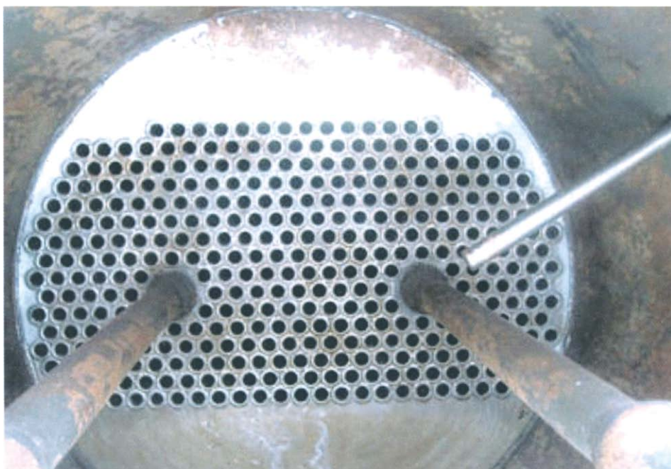
Fig. 24.6. Inside an acid cooler. Fig. 9.5 gives an external view. Tubes start through the tube 'sheet', shown here. They extend almost to the far end of the cooler where there is another tube 'sheet'. Cool water enters at this end and flows through the tubes to the far end. Between the tube 'sheets', the tubes are surrounded by warm acid moving turbulently around them. Heat transfers from the warm acid to the cool water (through the tube walls). The tube entering from the right contains a thermocouple. The polymer tubes in the foreground surround metal rods. The rods are bare between the tube 'sheets'. An electrical potential applied between them and the water tubes anodically protects the tubes against acid side corrosion.
