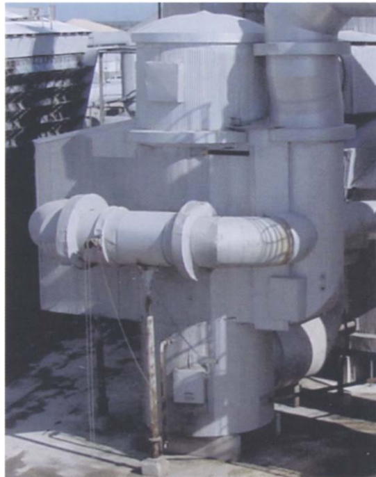
Fig. 22.2. Photograph of gas bypass flue around cross flow gas-to-gas heat exchanger. In this case, the amount of bypass is controlled by manually adjusting a butterfly valve in the bypass flue (note chain below the valve). In most cases, the valve is controlled automatically by a thermocouple placed just beyond the heat exchanger exit gas/bypass gas re-combination point.
