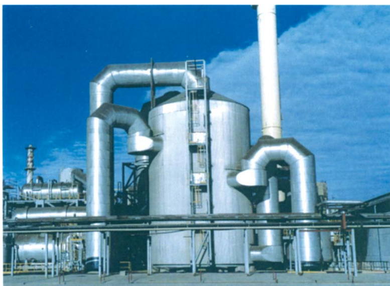
Fig. 7.7. Photograph of catalyst bed converter, courtesy Outokumpu OYJ www.outokumpu.com . Gas inlet and outlet flues are shown. Others are hidden behind. Fig. 7.6's gas coolers are also hidden behind. Converter walls and roofs are designed to be strong enough to withstand their acid plant's main blower 'shutoff' pressure without damage (Friedman and Friedman, 2004). Catalyst 'tray' supports are also strong enough to withstand the downward force exerted by the descending feed gas (at the converter's operating temperature).
