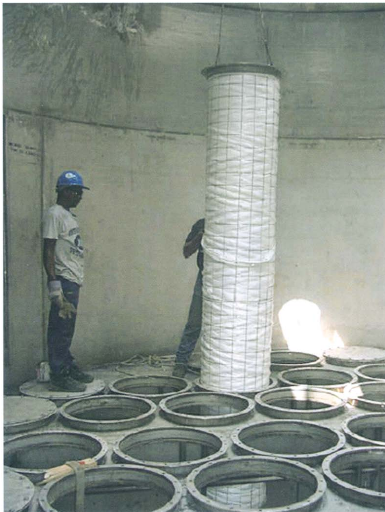
Fig. 9.3. Acid mist removal 'candle' filter being installed atop a stainless steel \text{H}_2\text{SO}_4 making tower. It is one of many. Exiting gas passes inward through the candle fabric and out the top of the candle – then out of the tower. The acid mist is caught in the candle fabric by impact, diffusion and Brownian forces (Brink, 2005; Friedman and Friedman, 2004; Lee and Byszewski, 2005; Ziebold and Azwell, 2005). The large total area of the candles gives a low gas velocity through the fabric, which allows 99+% capture of the mist. The captured mist trickles down the fabric and drips back into the tower or into collection pipes (Outokumpu 2005).
