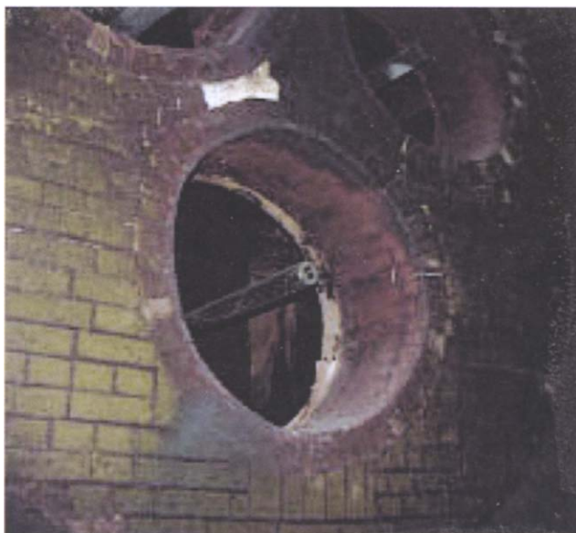
Fig. 3.3. Burner end of sulfur burning furnace. Atomized molten sulfur droplets are injected into the furnace through steam-cooled lances. Dry combustion air is blown in through the circular openings behind. The sulfur is oxidized to SO_2 by Reactions (3.1) and (3.2). Atomization is done by spiral or right angle flow just inside the burner tip.
