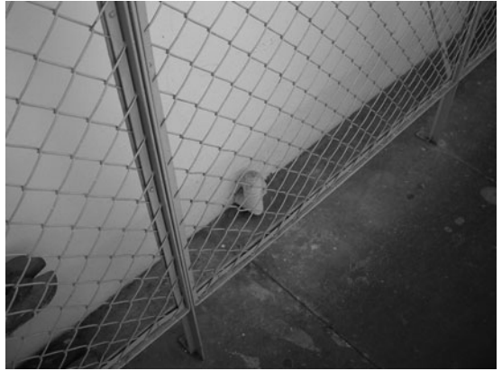
FIG 9.9 Now capped off, this pipe once supplied the gas to a wall covered with burners.
