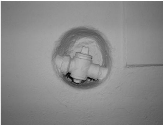
FIG 2.39 Main gas tap.
