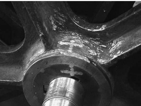
FIG 16.I2 Repairs using cold stitches can be clearly seen; these look like a row of filled holes.
