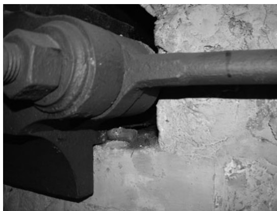
FIG 8.29 A roller below the foot of a bell frame standard.
