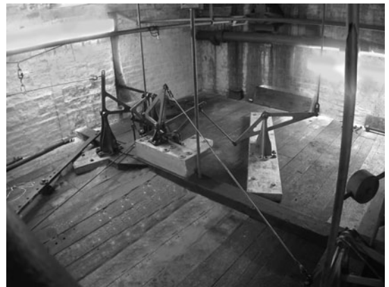
FIG 2.36 Inside the link room. The cluster of cranks is directly above the quarter train and the bar on the floor to the left holds the fly arbor bearings.
