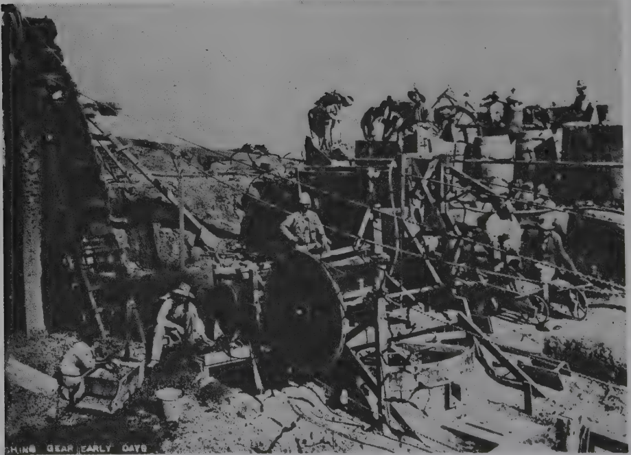
Fig. 4.22. Washing pans at the pipe mines in the early days operated by horse whims and later by steam.
