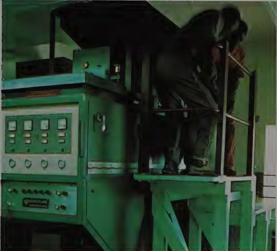
X-ray final extraction is common at the larger plants. This Sortex machine is one of several at the computer-controlled Consolidated Diamond Mines plant in Namibia.
