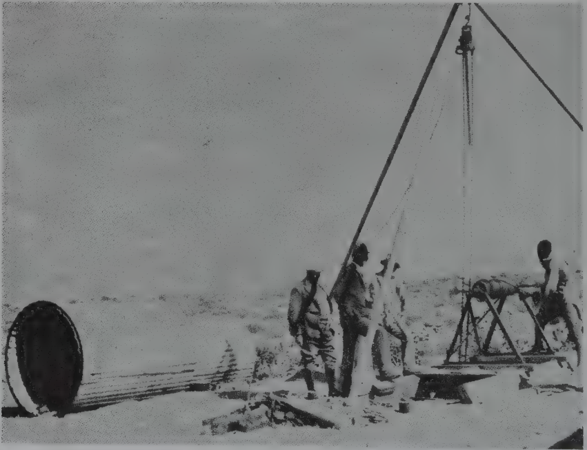
Fig. 3.27. The first shaft which was sunk through the sand on a marine terrace to the diamond-bearing gravels, on what is now the rich C.D.M. concession in Namibia (South West Africa).
