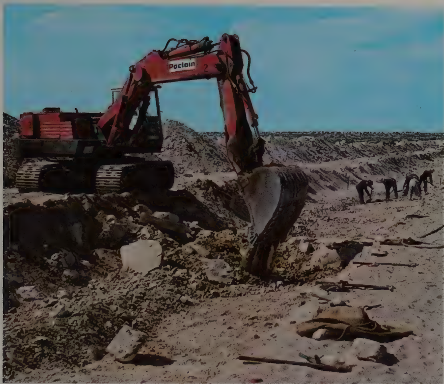
After inspection pits have been dug in a row and sampled, a trench is opened up, preparatory to alluvial mining. A Poclair digger works on this one in Namaqualand.
