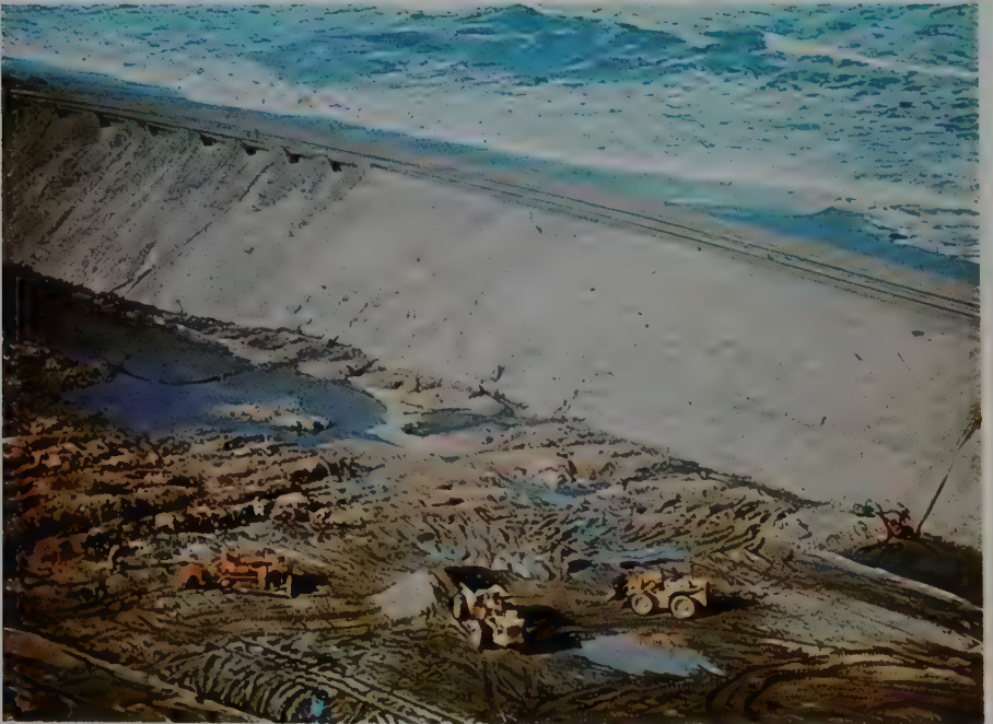
The area inside a paddock along the tidal strip is pumped out and the over-burden removed before it can be stripped of the diamondiferous gravels, which go to the treatment plant.
