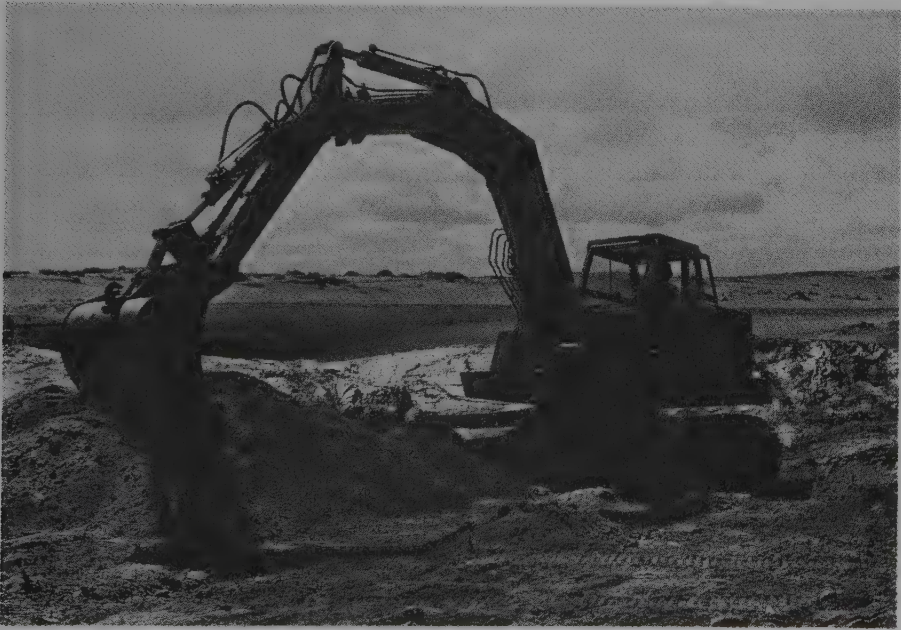
Fig. 4.41. A Poclair trench digger, used to clear deep gullies and also to make prospecting trenches and to load sample boxes.
