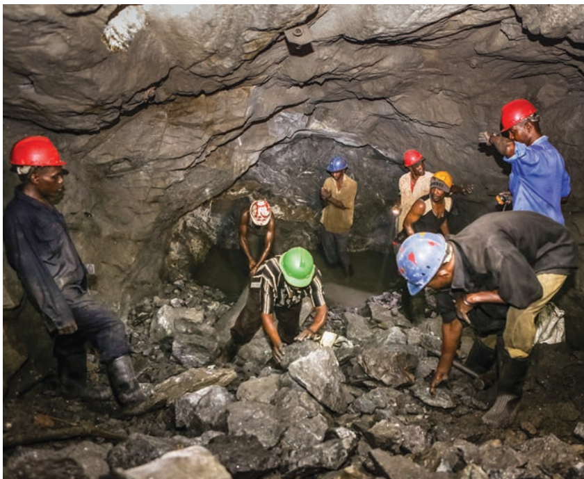
Figure 31: Miners sort through waste rock at the working face of Scorpion mine tunnel No. 4. The ceiling in this area has been reinforced with split-sets. Photo by Louis Brunet.
