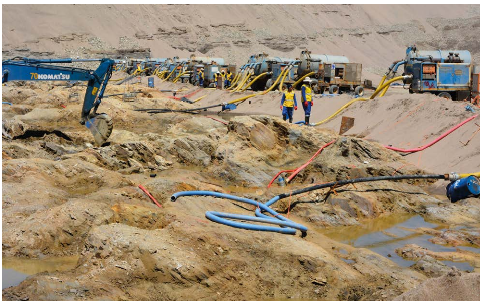
Figure 22: A portion of the exposed bedrock (right side) has been vacuumed to remove any diamond-bearing sediments, while on the left an excavator prepares the area for the transvac crews. Photo courtesy of Namdeb.
