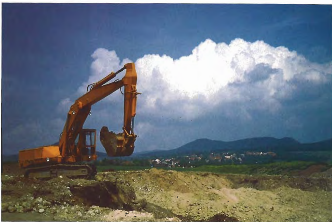
Figure 3. A power shovel is used to remove the overburden and garnetiferous gravels at Podsedice. In the background can be seen remnant pipes of Tertiary volcanism in the Bohemian Hills. Photo by J. Schlüter.
