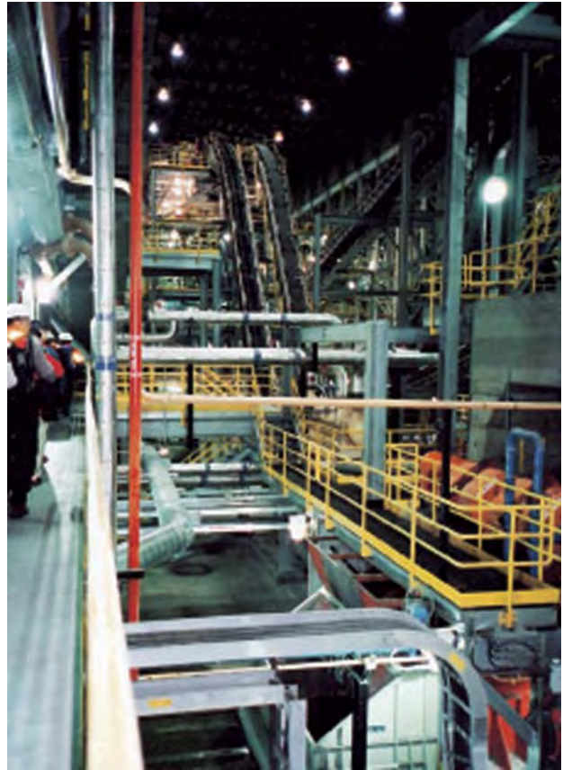
Figure 4. The high-angle conveyor belts in the top of this image carry diamond ore to the gravitational separators at the Diavik processing plant. The ore cannot be seen because it is covered by a second rubber belt. Photo by Mary L. Johnson.
