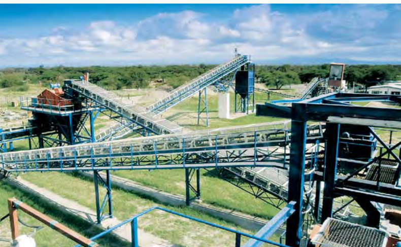
Figure 34. This customized processing plant has been converted by AFGEM from a former graphite plant to extract tanzanite. This photo, taken from the dense media separation area, shows a network of conveyor belts that eventually routes material to the sort house (far right), where it is hand-picked under stringent security measures. Photo by Reyno and Claire Scheepers.
