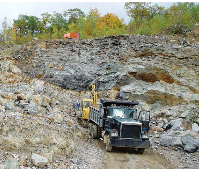
Figure 7. An excavator and dump truck are used to remove mined material from the open cut at Mt. Mica, as shown in this October 2004 photo by Gary Freeman.
