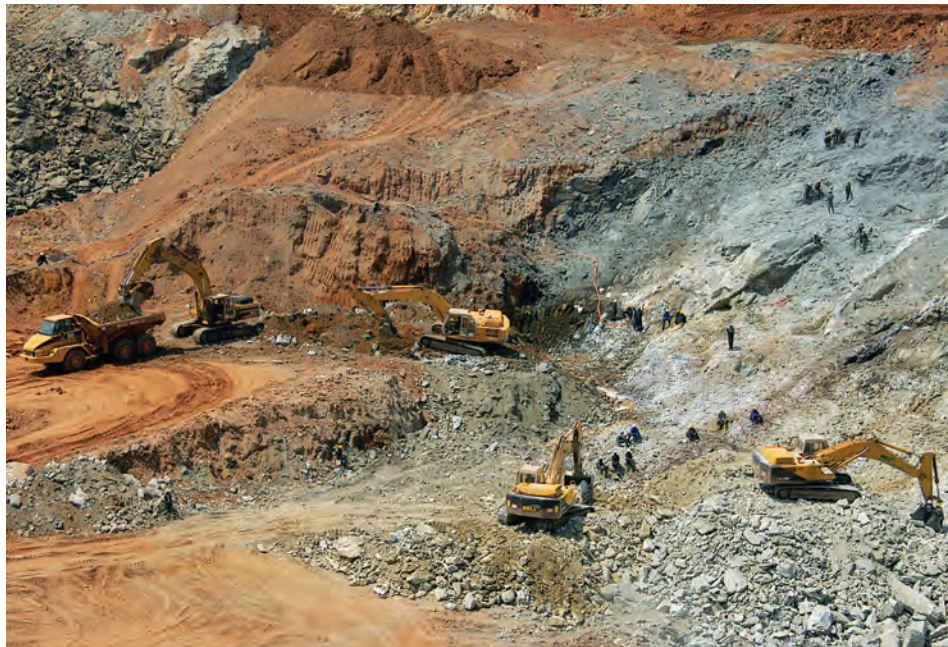
Figure 5. The Grizzly mine employs large earth-moving equipment in a highly mechanized operation. The excavators used in the Kafubu emerald mines typically weigh 25–30 tons and have a bucket capacity of approximately 1.6 m 3 . Photo by B. M. Laurs.
