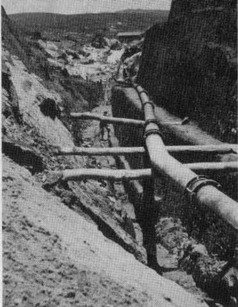
• Canal cut through decomposed basic igneous rock, separating massa outcrop at Daltas Mine
