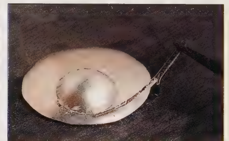
Solder is applied to a joint using a soldering stick. Note how the paillon is in place to indicate flowing temperature.
