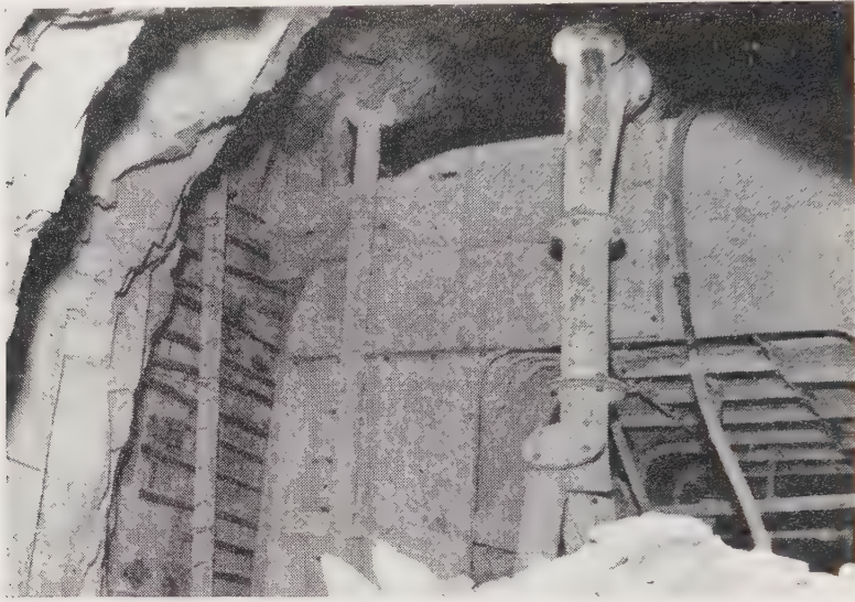
Fig. 11—View of shuttering and concrete delivery pipe. Side packing can also be seen
