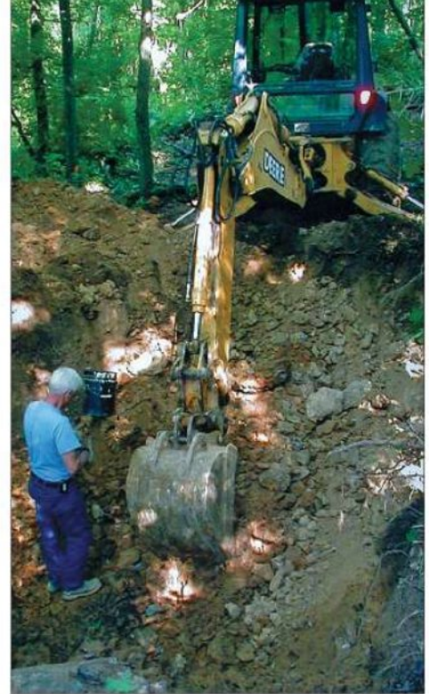
Roy and his backhoe have dug a number of pits, showing plenty of exposed flint, at the Nethers Quarry site.
